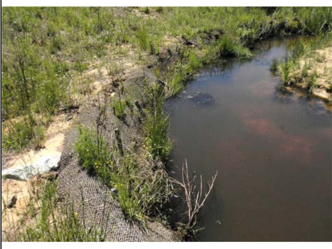
Stream Problem Area 1 (lack of woody vegetation establishment along left bank), R2 Station 32+25
