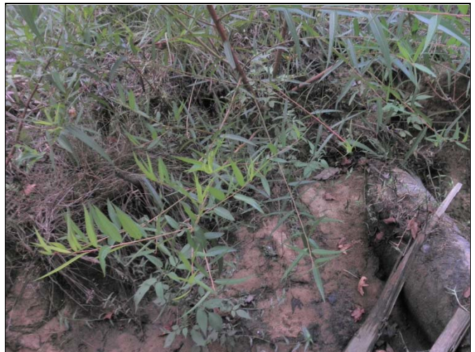
Reach 2: Station 40+50, bank stabilization work (livestakes shown here were planted in January 2017)
