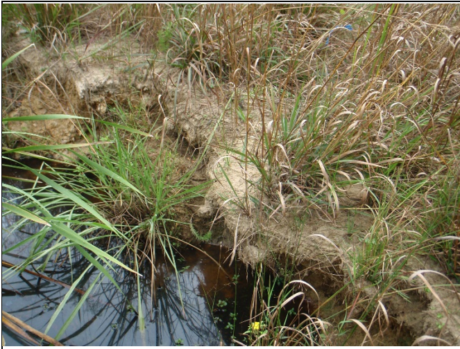
SPA-1: Bank scour and damaged livestock establishment from Hurricane Florence, left bank of R2, Station 34+75
