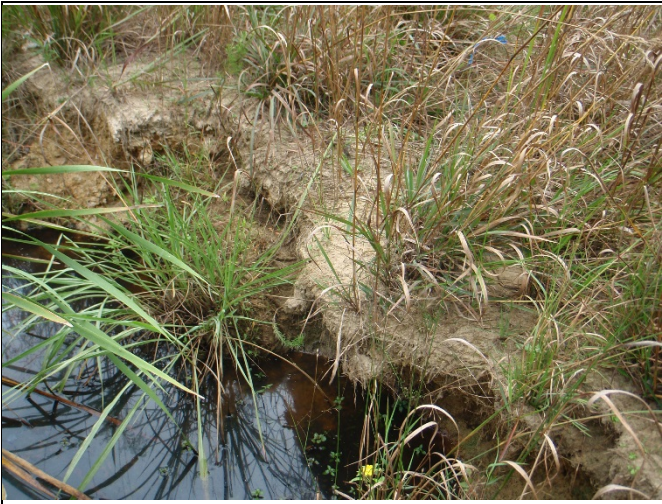
Previous bank scour from Hurricane Florence, left bank of R2, Station 34+75 (BEFORE)
