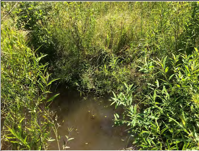
R2 Station 35+75: Previous bank repair on left bank from Hurricane Florence scour (photo: June 2020)
