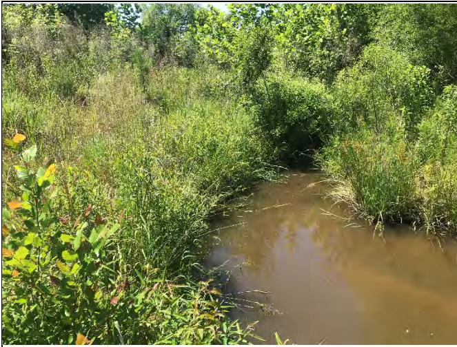
R2 Station 34+75: Previous bank repair on left bank from Hurricane Florence scour (photo: June 2020)
