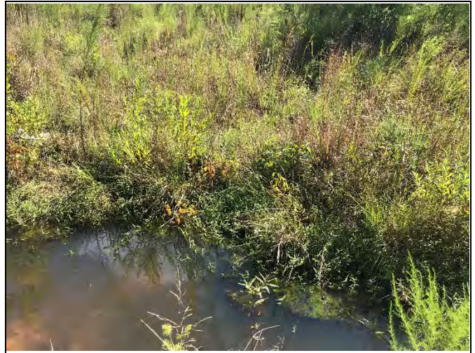
R2 Station 35+75: Previous bank repair on left bank from Hurricane Florence scour (photo: October 2020)
