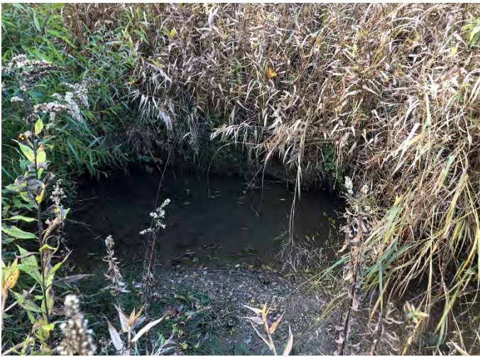
Photo 3 – UT1 R1: Station 202+90-203+15 – Left Bank Scour. 10-26-2021
