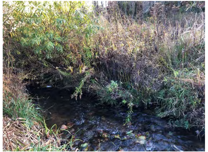
Photo 2 – Vile Creek R1: Station 103+90-104+20 – Right bank scour. 10-26-2021
