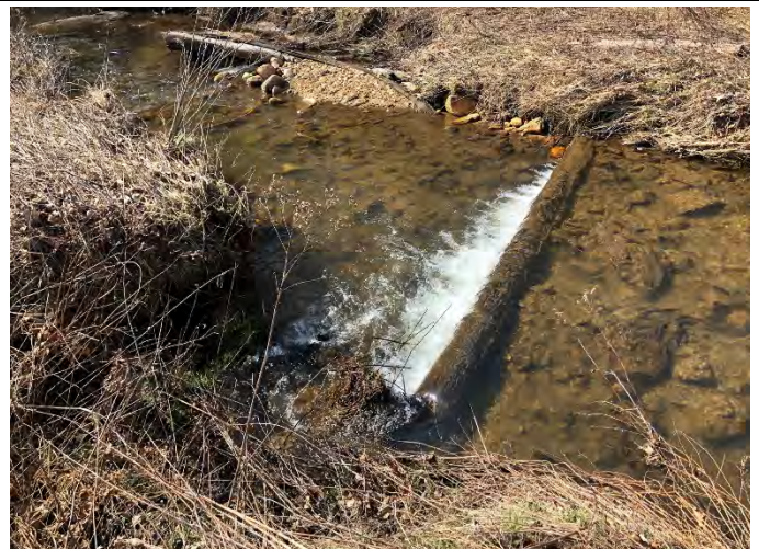
Vile Creek R2: STA 122+20-123+00 – Left Bank Erosion 3-17-2021
