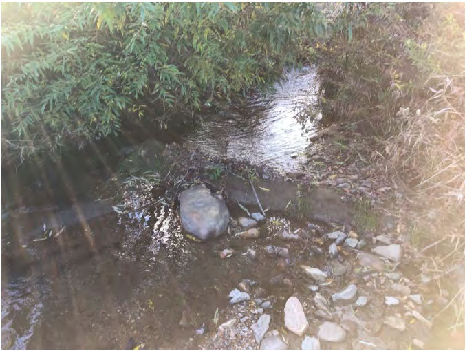
Photo 1 – Vile Creek R1: Station 103+90 – Right bank piping and scour around log sill. 10-26-2021
