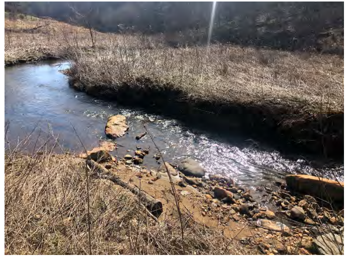
Vile Creek R2: STA 118+80 – J-Hook structure failure 3-17-2021
