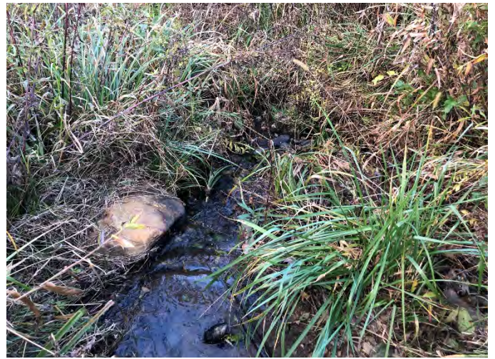
Photo 4 – UT1 R1: Station 204+90 – Structure missing. 10-26-2021
