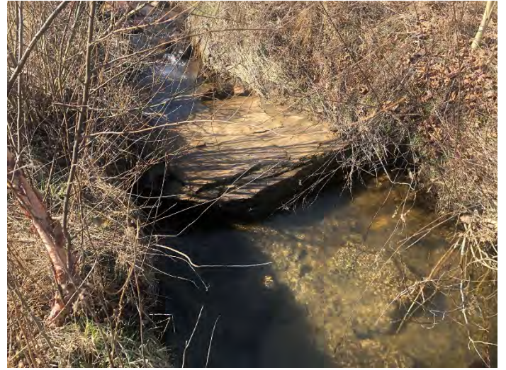
Photo 8 – UT1 R2: Station 220+98 – Piping around structure 3-17-2021
