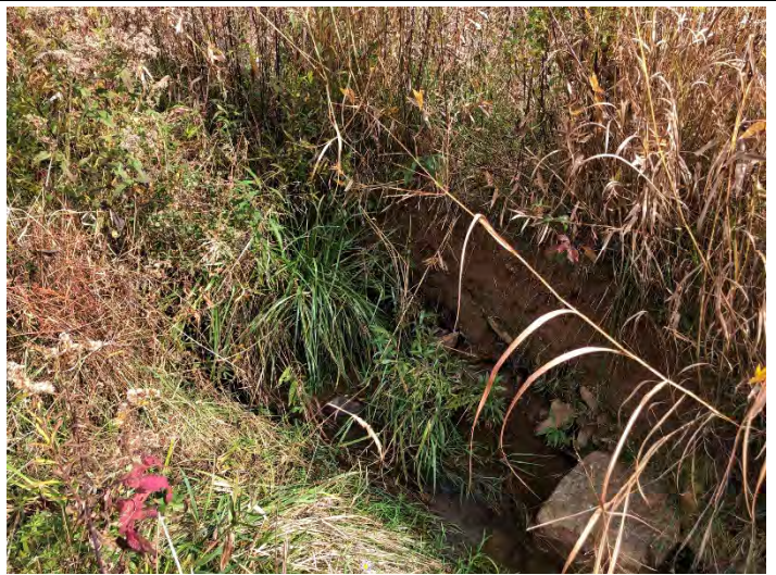
Photo 10 – UT2: Station 305+00 – 305+50 – Bank scour. 10-26-2021
