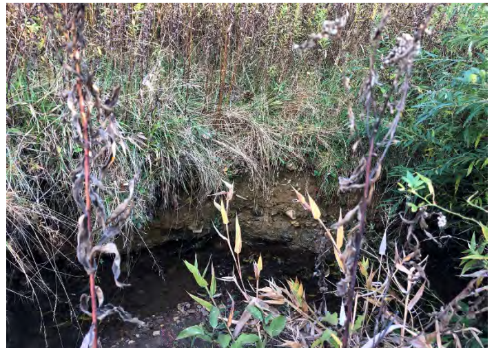
Photo 6 – UT1 R1: Station 206+40 – 206+60 – Bank Scour 10-26-2021
