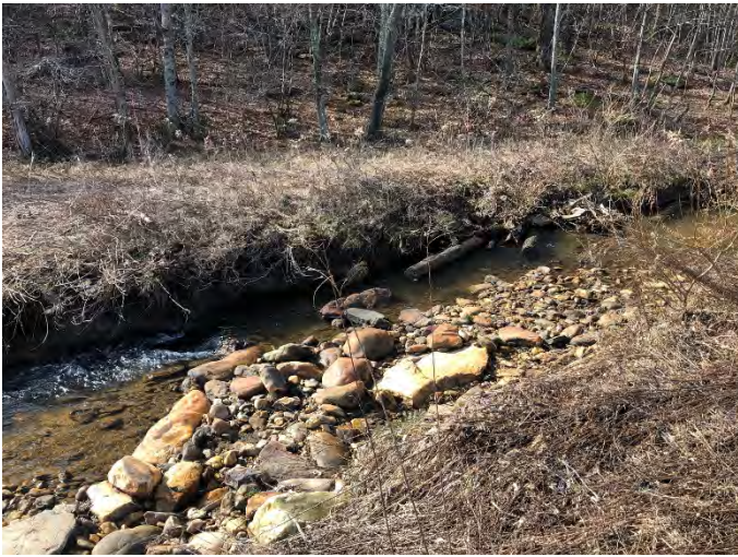
Vile Creek R2: STA 118+50 - 118+80 - Right Bank Erosion 3-17-2021
