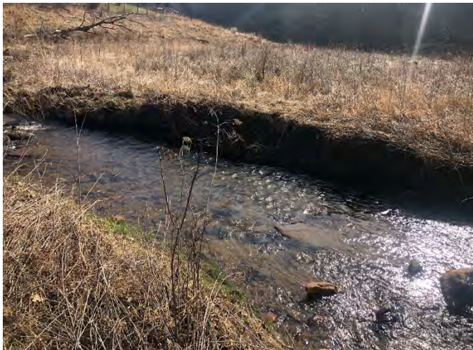
Vile Creek R2: STA 120+70 - 121+00 – Right Bank Erosion. 3-17-2021
