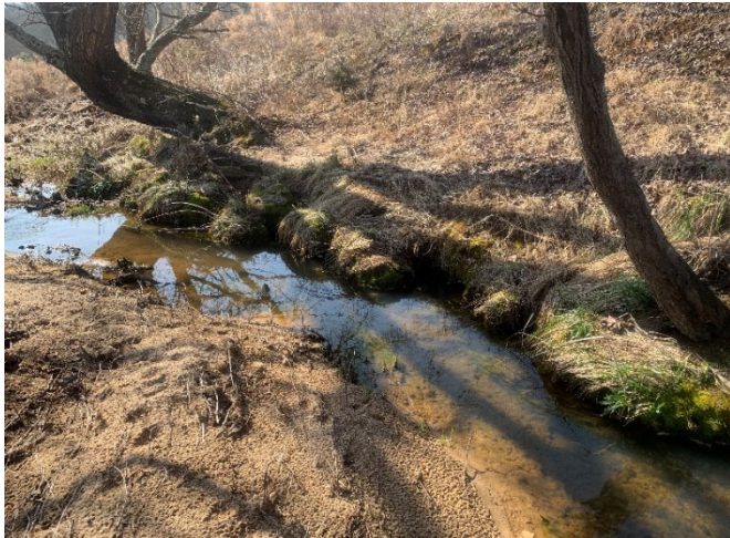
UT1 R2 Right Bank Erosion (STA 121+00-121+15) – view downstream (2/9/2021)
