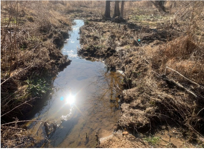
UT1 R2 Right Bank Erosion (STA 120+00-120+20) – view downstream (2/9/2021)
