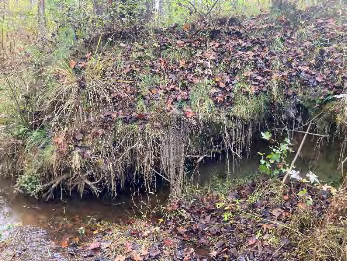
Elliott Creek Bank Scour (STA 141+30) – view downstream (11/5/2021)
