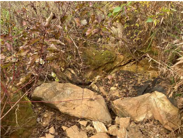
Royster Creek R1 Rock Sill Failed (STA 806+74) – view upstream (11/3/2021)
