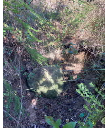
Scott Creek Channel Incision (STA 1211+25 – 1211+36) – view upstream (10/27/2021)
