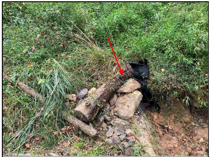
UT4-R1b, SPA #3 Bank Repair (Scour filled-in with soil, matting and rock/logs installed on top, Sept. 2021)
