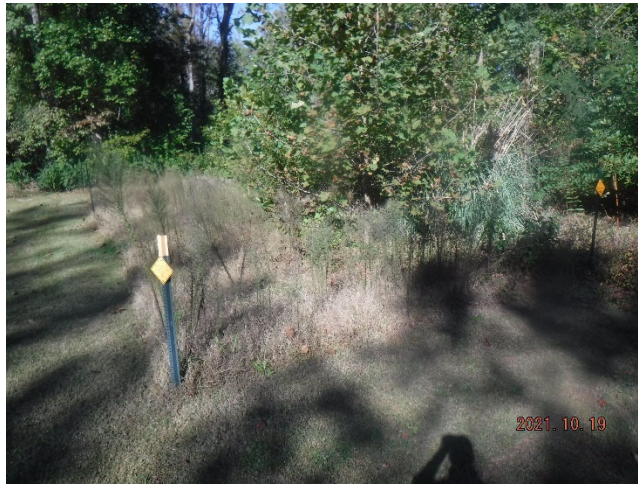
Candy Creek Reach 3 - Easement encroachment at Hopkins Road, LB (Sta. 149+00-150+00) (10/19/2021)
