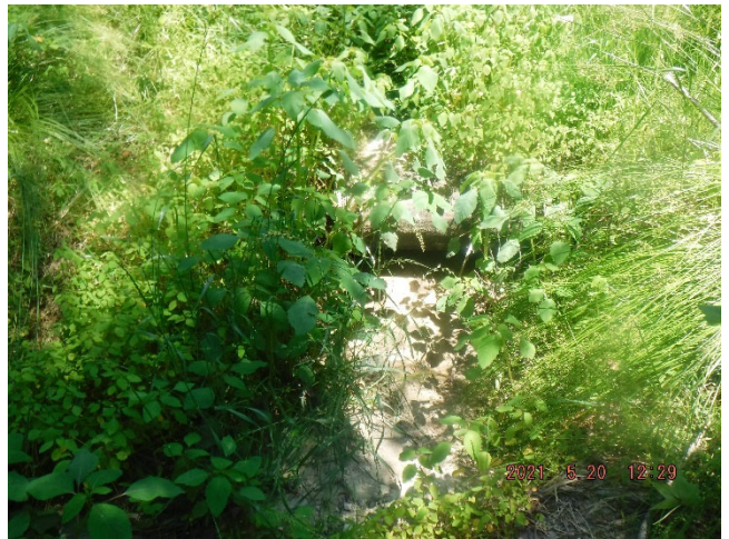
UT1D - Failed structures (Sta. 253+00) (05/20/2021)
