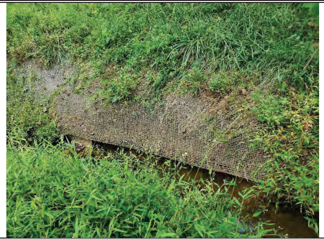
Figure 5.14 Minor erosion at removed crossing of UT MC (9/7/2021)
