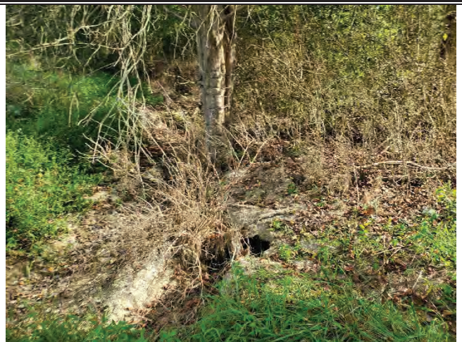
Figure 5.12 Minor Erosion culvert crossing UT2 (9/7/2021)
