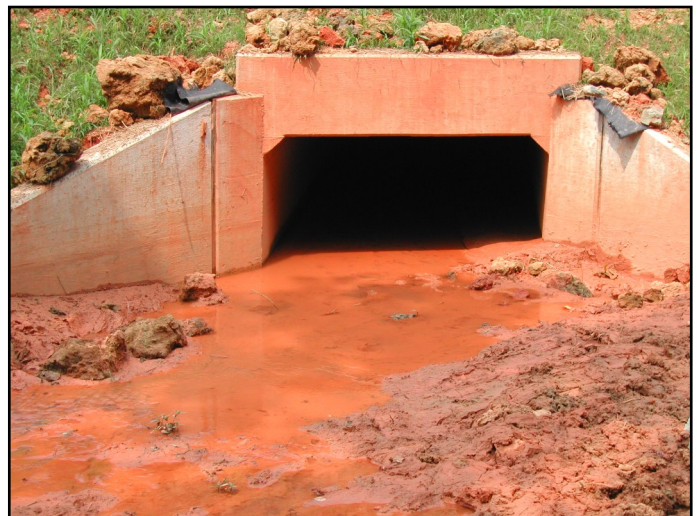
Uncontrolled sediment discharges from an abandoned construction site led to heavy sediment deposits in a stream and culvert. Photo Credit: Rich McLaughlin.
