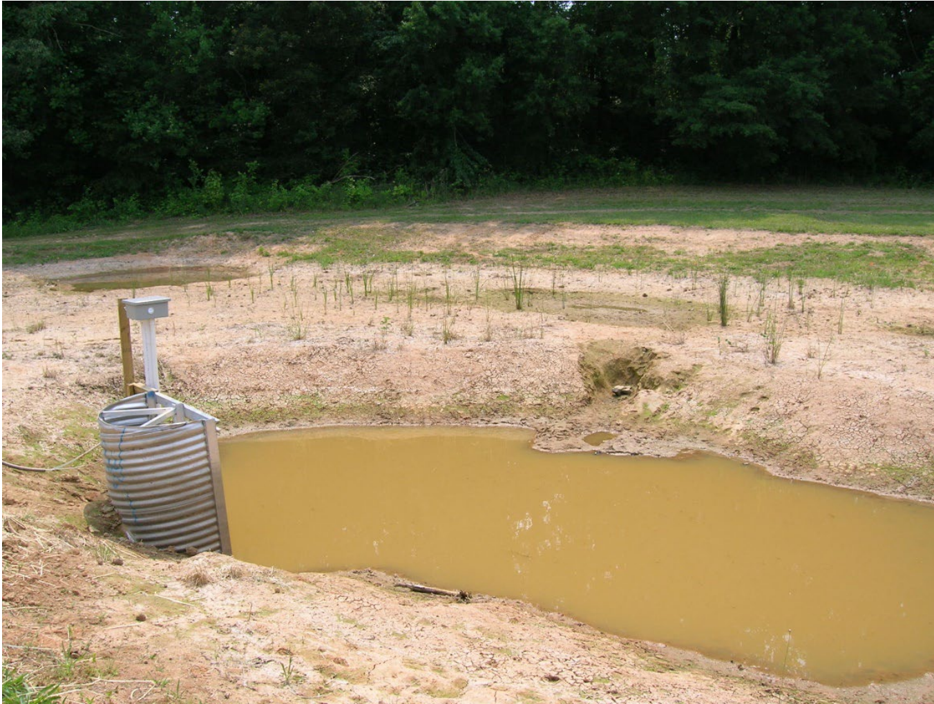
one cell of an experimental 3-tiered stormwater wetland in need of maintenance
