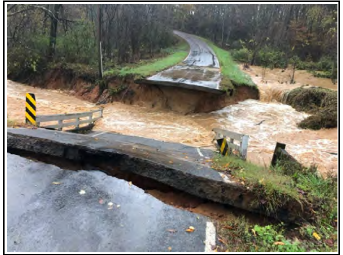
Flooding from Zeta remnants collapsed the bridge immediately upstream of R7 (10/29/20)
