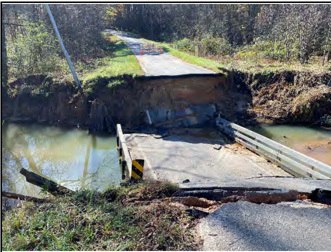
The bridge after the flooding subsided (11/4/20)
