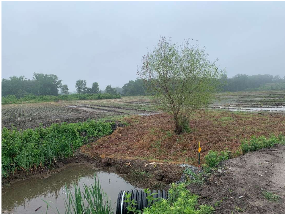
Ditch Plug Constructed at NE corner of the Site (view SW) – taken 5/25/2022
