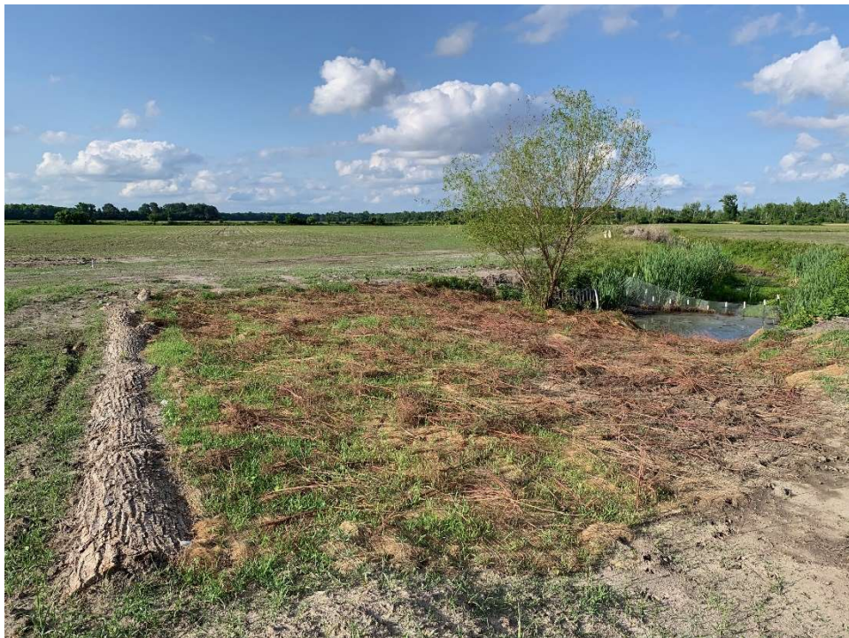
Ditch Plug Constructed at NE corner of the Site (view NE) – taken 5/25/2022
