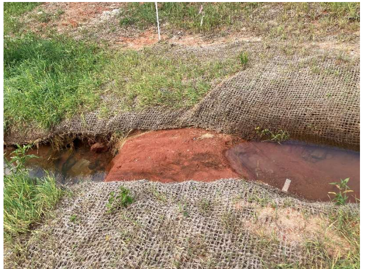
Displaced Riffle Material – UT1 Reach 1 STA 211+20 (06/01/2022)
