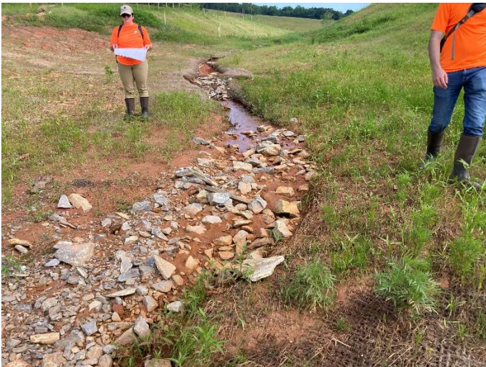
Displaced Riffle Material in Pool – UT1 Reach 1 STA 212+75 (06/01/2022)
