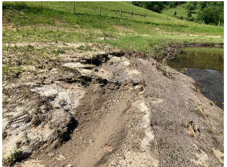
Floodplain Scour behind Top of Bank – NL Hunting Creek R1 STA 102+60 (06/01/2022)
