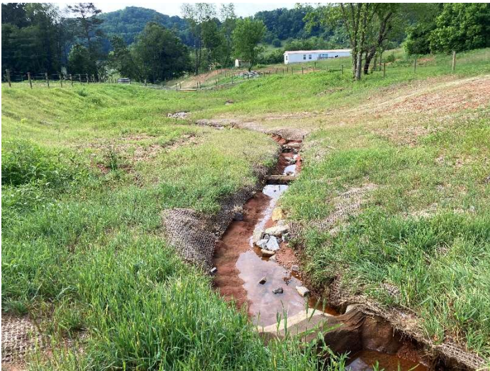
Displaced Riffle Material – UT1 Reach 1 STA 210+50 - 212+50 (06/01/2022)
