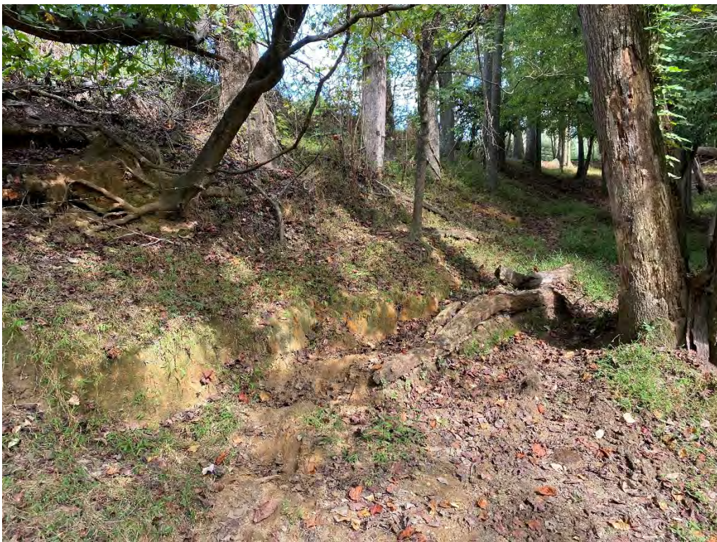
Photo 10: Erosion along eastern abutment contact.
