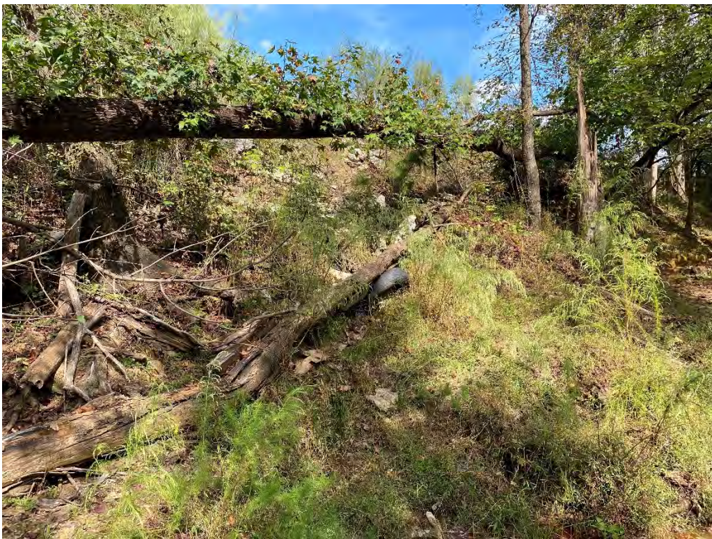
Photo 14: Concrete spoils and tires used in previous dam repair attempt.
