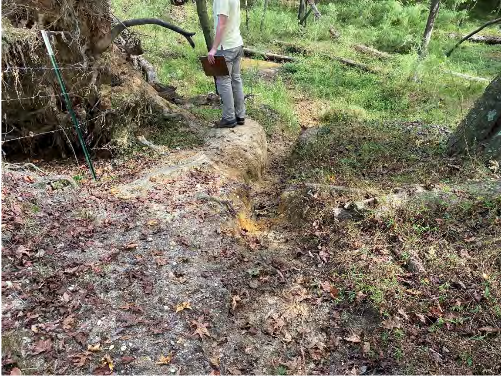
Photo 9: Shallow gully along western abutment contact.
