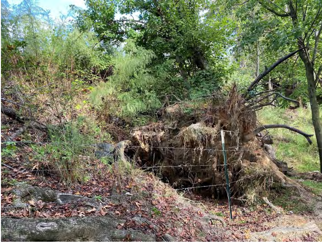
Photo 7: Uprooted tree on downstream face has removed portion of dam embankment.
