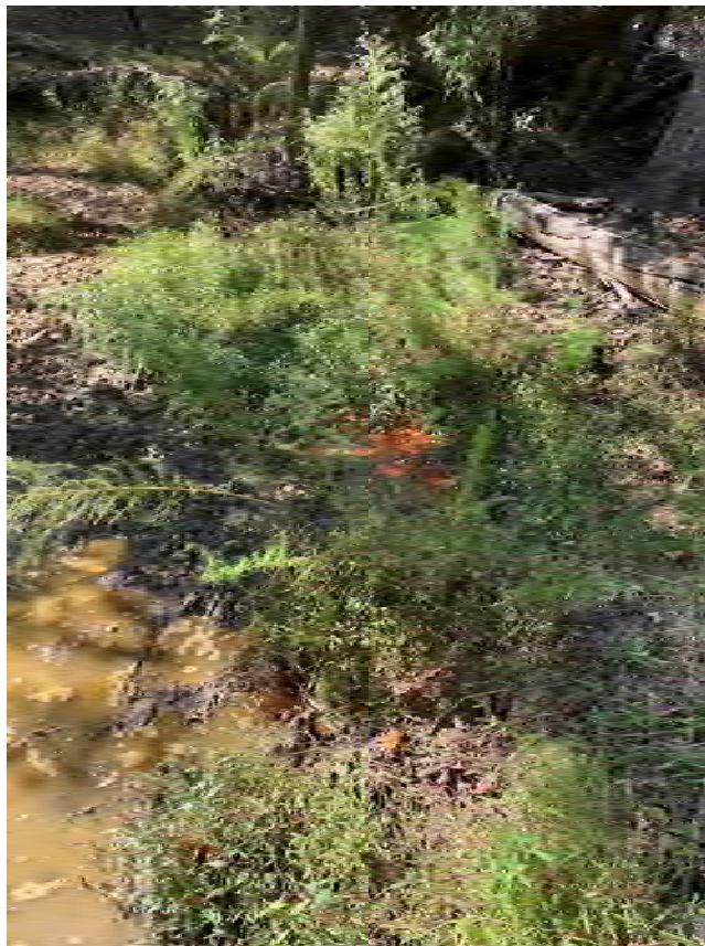
Photo 12: Pondered water beneath downstream toe of dam.
