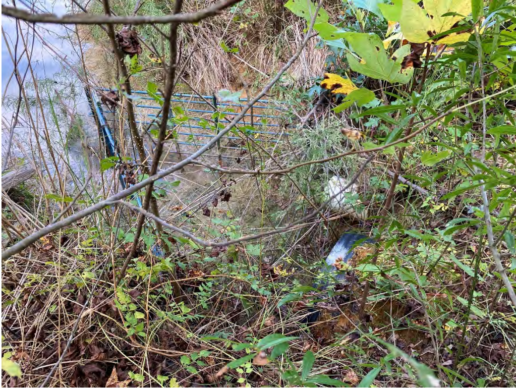
Photo 15: Upstream intake of 24" HDPE culvert and 8" PVC pipe with triangular trash rack.
