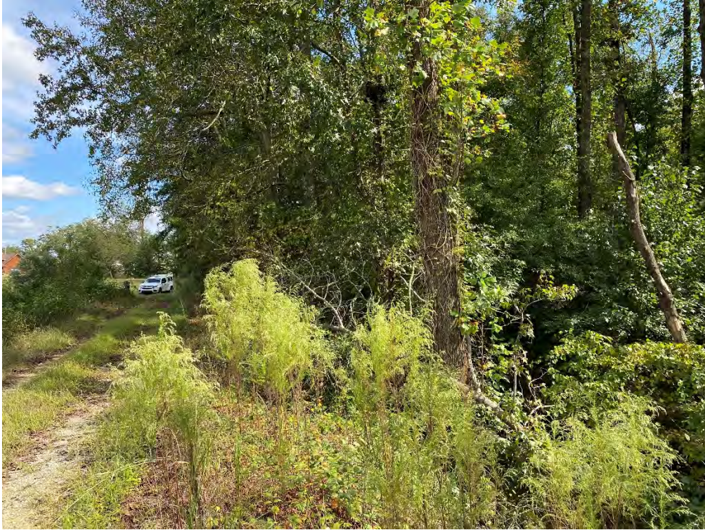
Photo 5: Downstream face heavily vegetated by trees, looking east.
