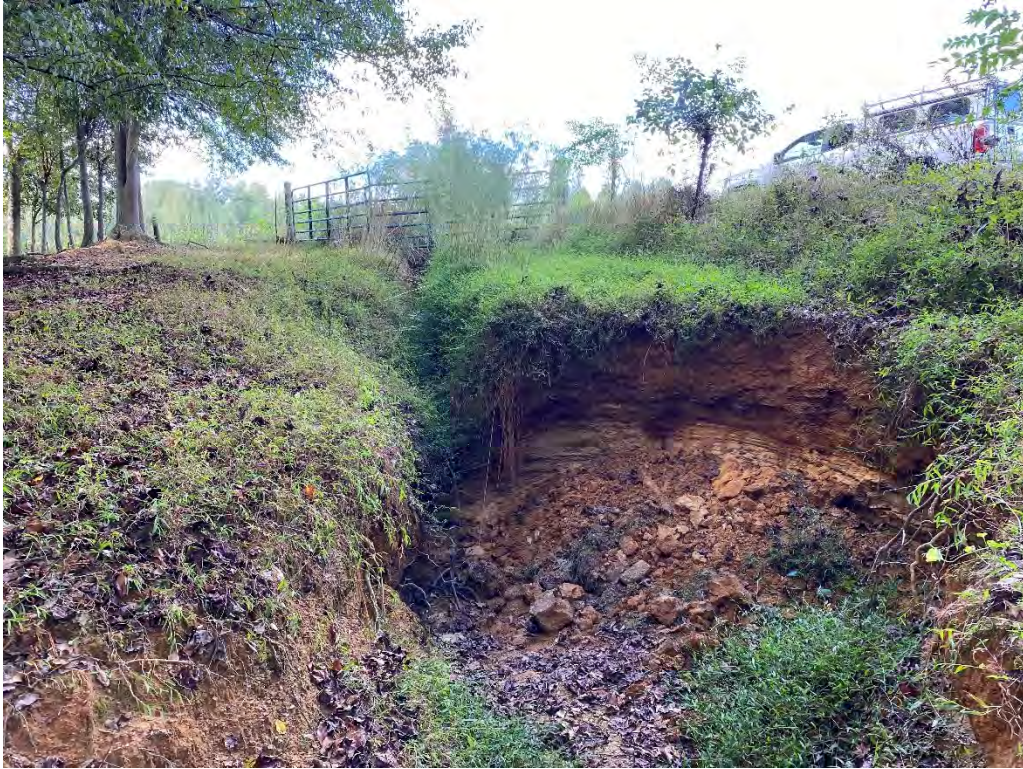
Photo 17: Headcut of 6-8 feet in depth forming about 10 feet downstream of outfall.
