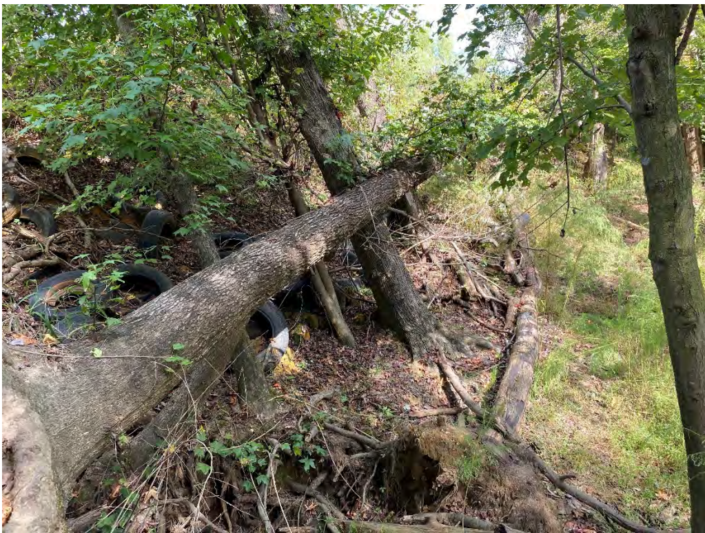
Photo 8: Uprooted tree on downstream face of dam in area of previous repair using tires and other refuse.
