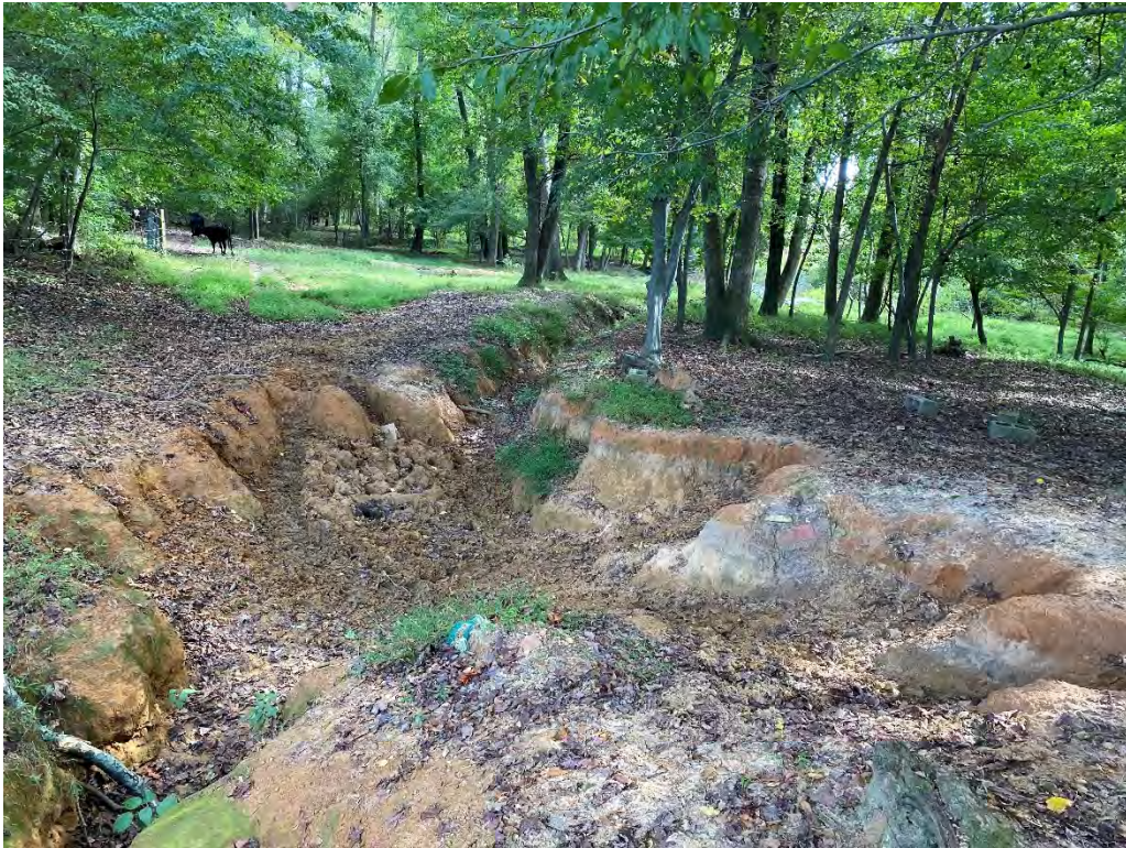
Photo 18: Cattle cross large gully immediately downstream of headcut.
