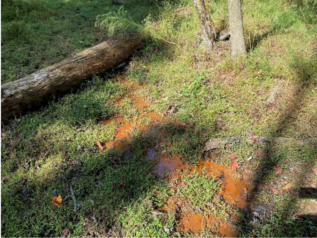
Photo 11: Rust-colored water ponding below downstream face due to seepage through dam embankment.
