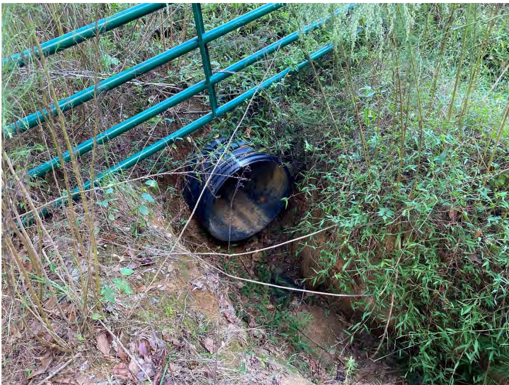
Photo 16: Downstream outfall end of 24" HDPE culvert with no 8" PVC pipe visible. Erosion directly beneath outfall continues downstream.
