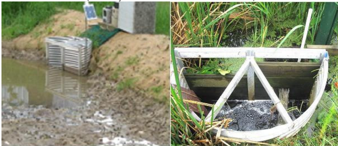
Figure 9-9 Outlet Structures with Flashboard Riser for Maintenance (Courtesy NC State Science House and BAE)
