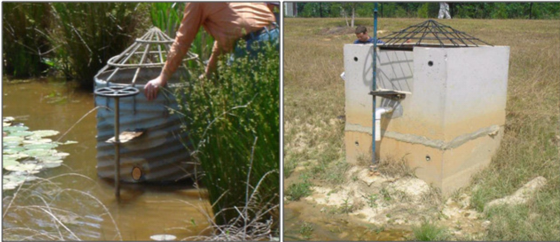
Figure 9-8 Outlet Structures with Manual Drawdown Valve for Maintenance
