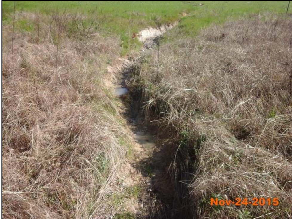
Project Reach 1 – Ditch/ Bare Area 20+75 Right Descending Bank
