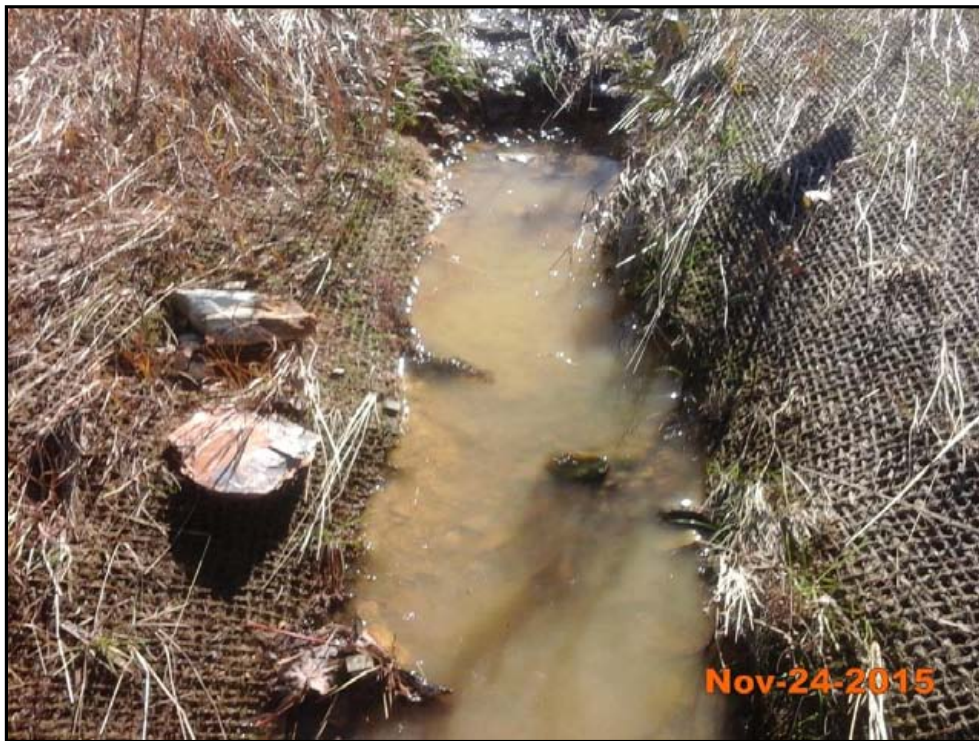
Project Reach 1 – Headcut/ Degradation 9+25
