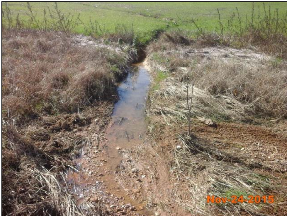
Project Reach 1 – Ditch/ Bare Area 12+00 Left Descending Bank
