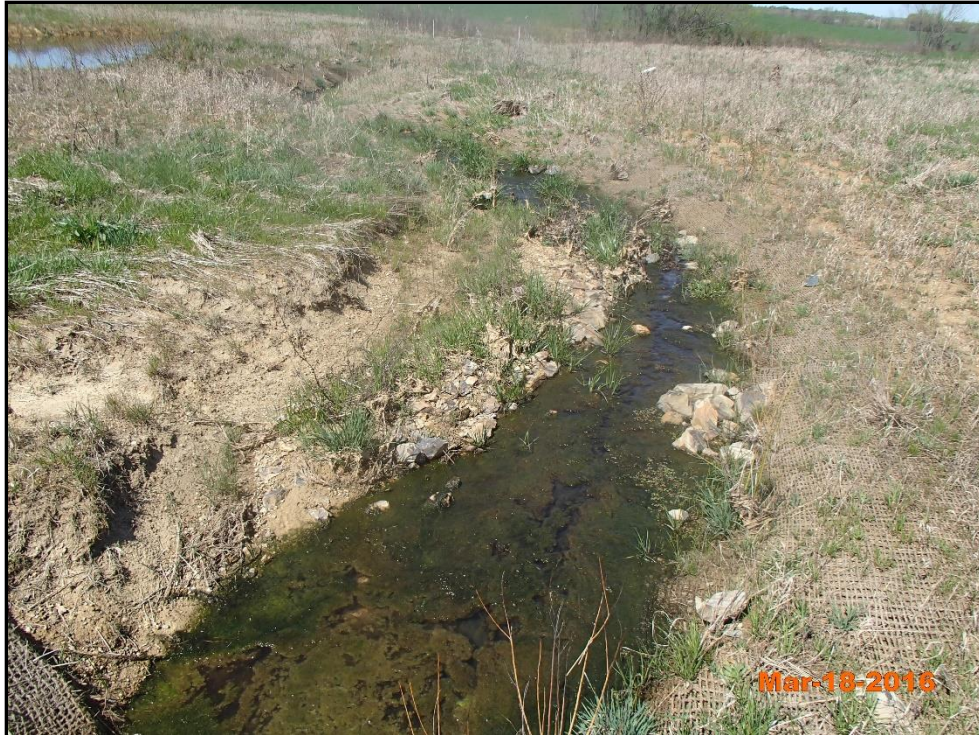
Project Reach 1 – Bank Erosion 9+50 Left Descending Bank
