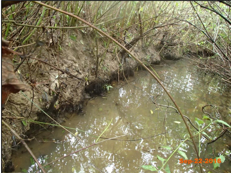
Project Reach 2 – Bank Erosion 11+25 Left Descending Bank
