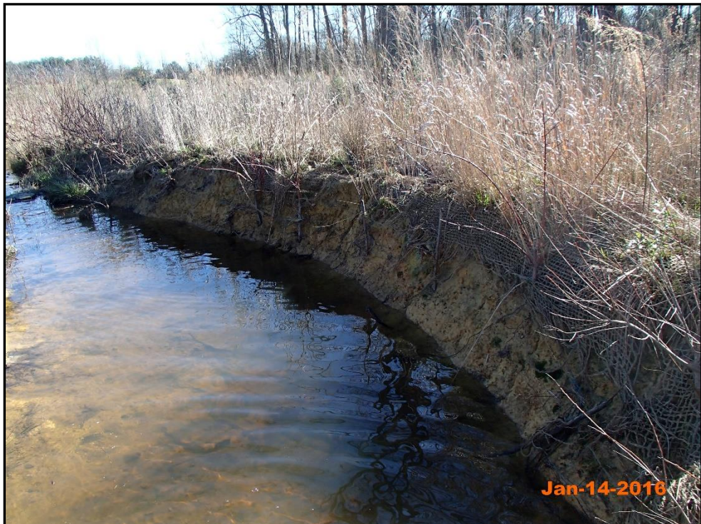
Project Reach 2 – Bank Erosion 22+50 Right Descending Bank
