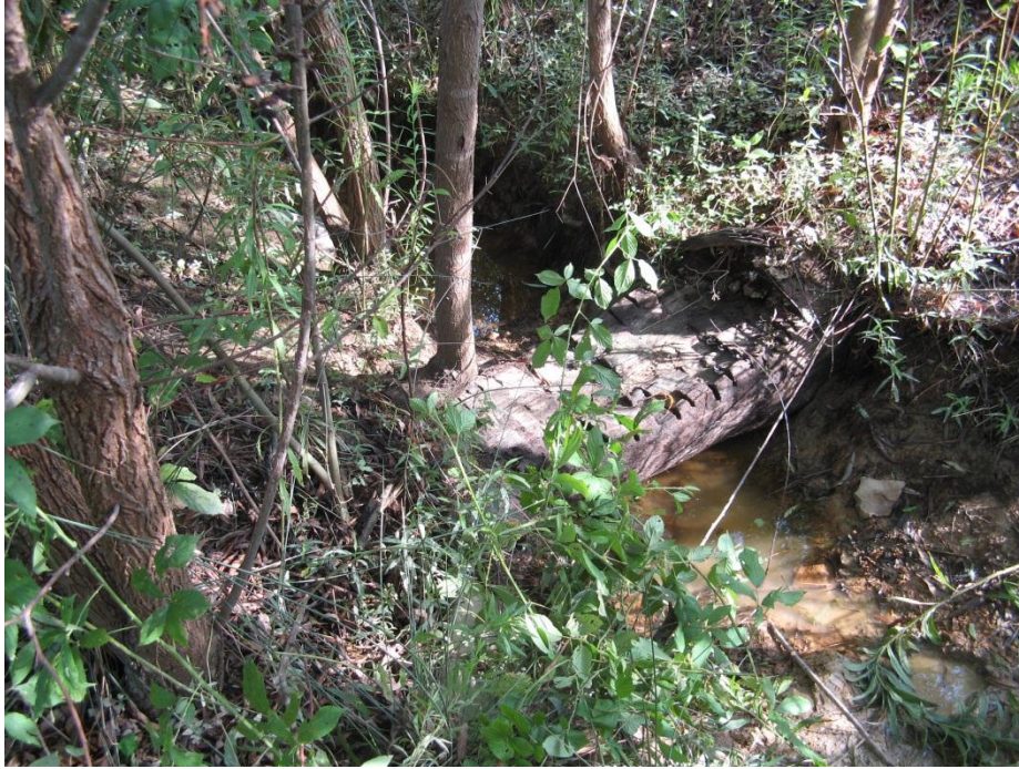
MY4-PA6 – failed sill log (photo from MY4 2011)
