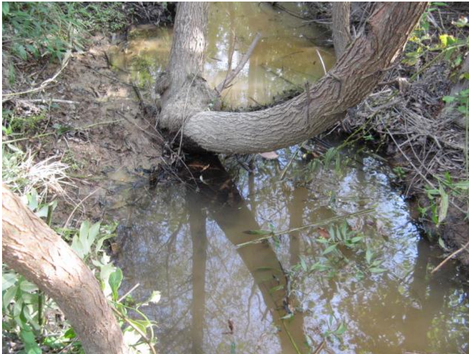
MY4-PA12 Channel obstruction
