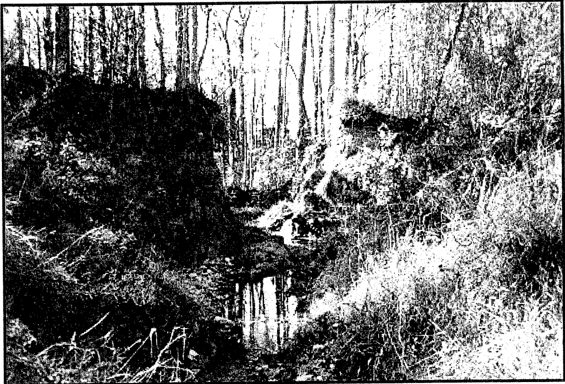
7. Breached center of dam wall. (Downstream View)
