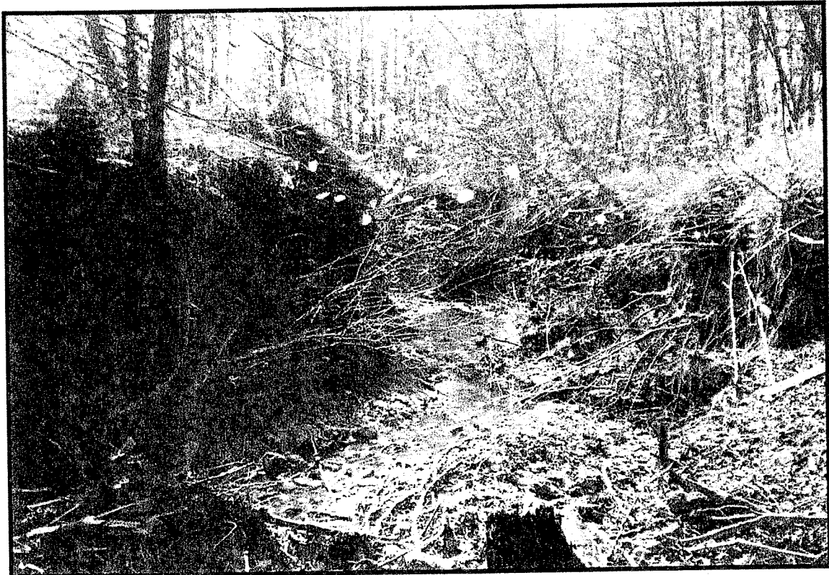
6. Severe down cut, resulting in vertical banks and loss of bank vegetation.
