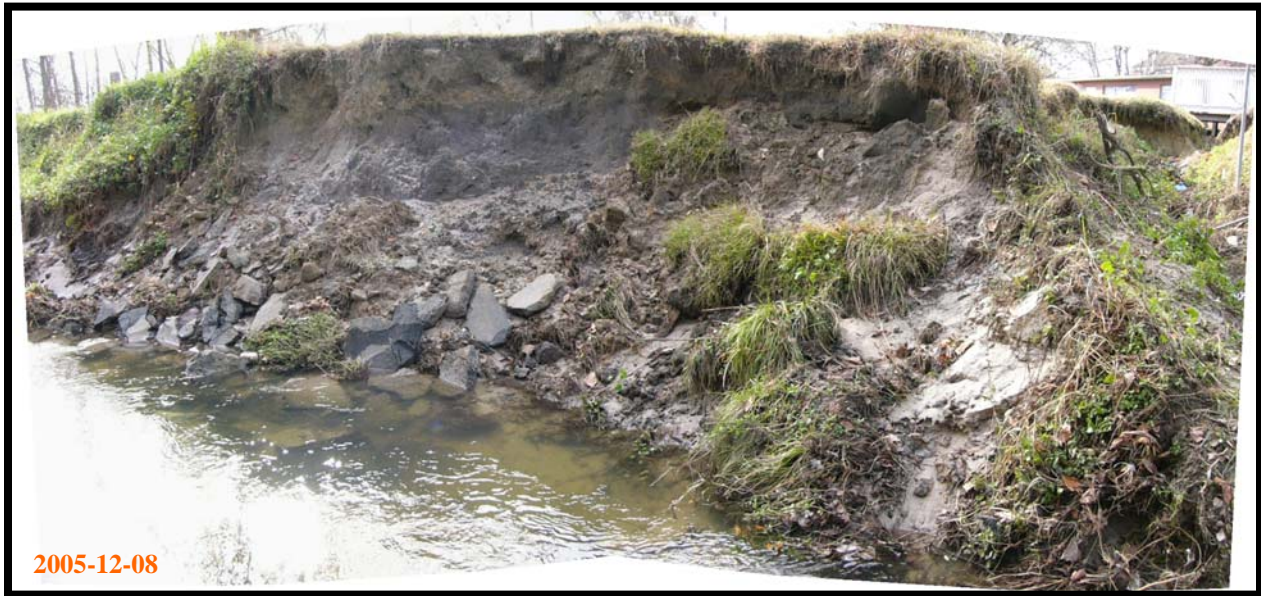
Erosion along Adkin Branch Banks - Looking Downstream
