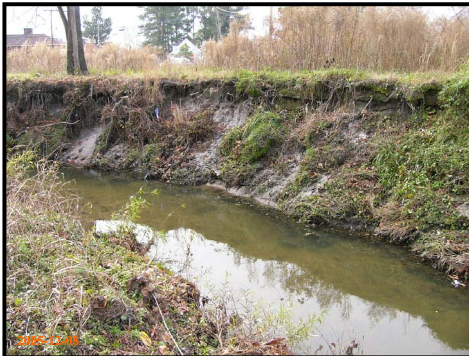
Erosion along Adkin Branch Banks - Looking Downstream
