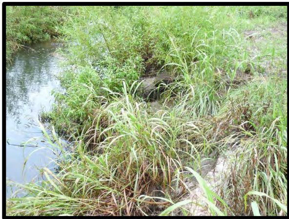
3.22 Moderate erosion near 71+50
