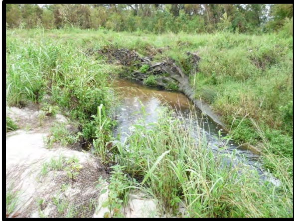
3.23 Minor erosion near 76+75
