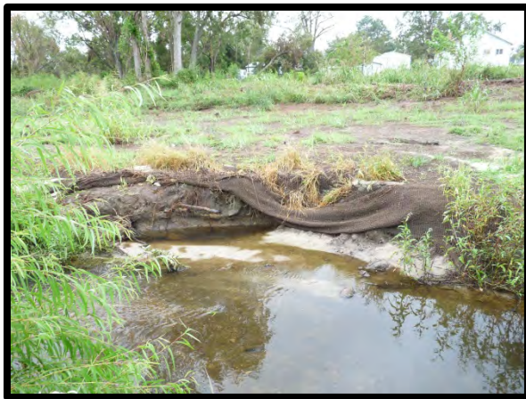
3.21 Severe bank erosion near 65+50
