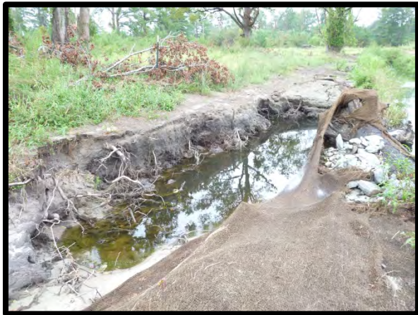
3.29 Severe erosion near 87+50
