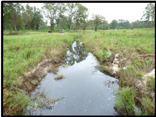
3.27 Moderate erosion near 84+25
