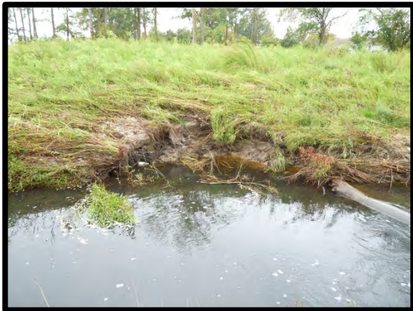
3.28 Moderate erosion near 85+80
