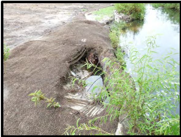
3.30 Moderate erosion near 91+50
