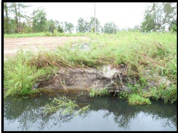
3.24 Moderate erosion near 81+10
