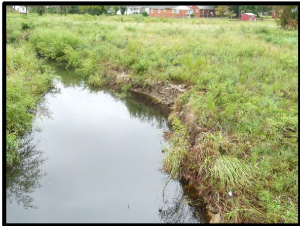
3.26 Moderate erosion near 83+50
