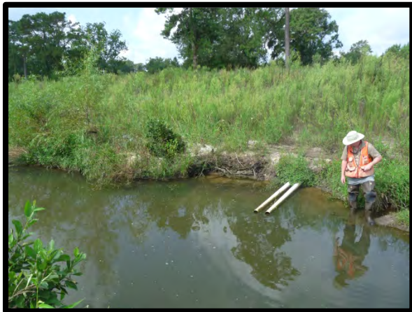
3.25 Severe erosion near 92+50
