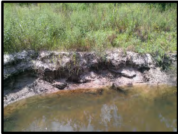
3.21 Severe bank erosion near 65+35
