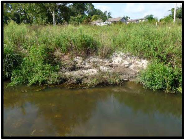
3.22 Severe erosion downstream of pedestrian bridge (84+30).
