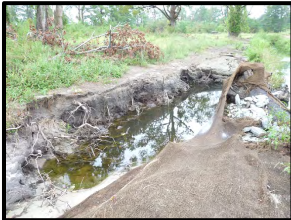
3.29 Severe erosion around vane arm 2011 (87+50)
