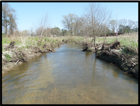
3.30 Scouring at XS 11
