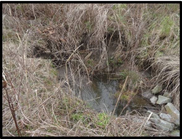
3.22 Scour in ditch off Elm Street near 44+50
