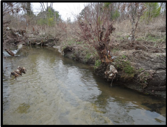
3.25 Minor and major erosion near 51+90
