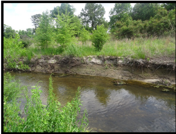
3.35 Severe erosion near 78+50
