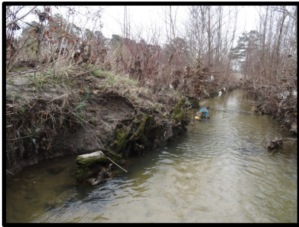
3.21 Minor erosion near 41+75
