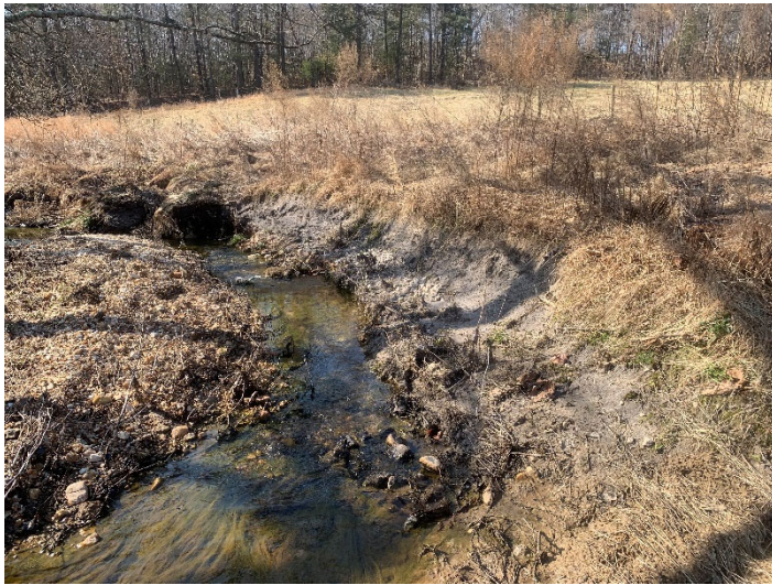
UT1 R2 Right Bank Erosion (STA 126+00-126+20) – view downstream (2/9/2021)
