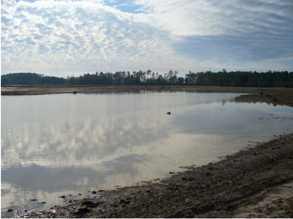
Photo 7. December 18 th - restored swamp run after 3” rain, three weeks after completion of construction.
