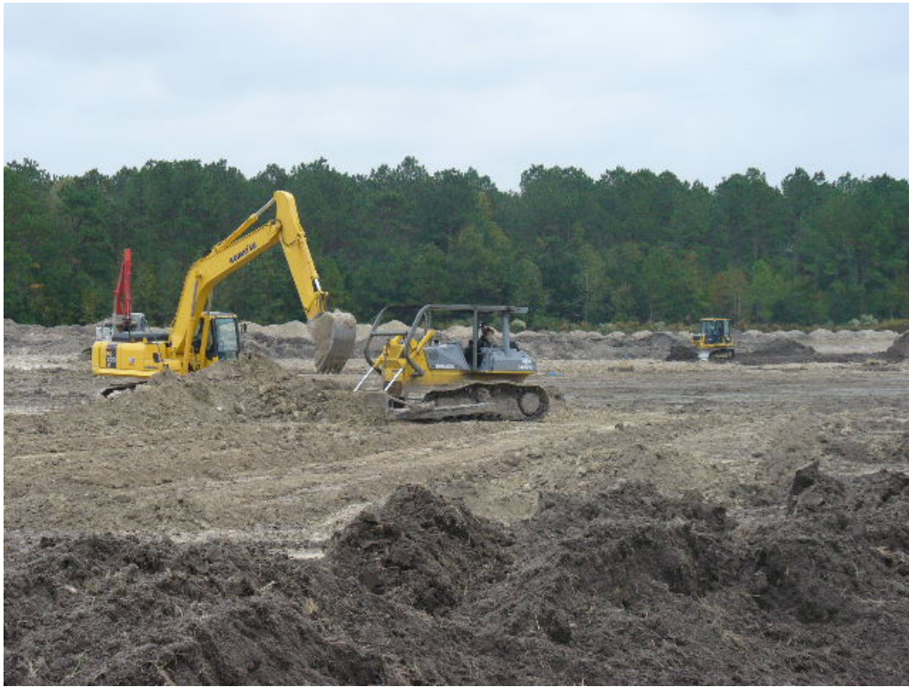
Photo 5. Redistribution of topsoil and final grading of restored swamp run and riverine wetlands.
