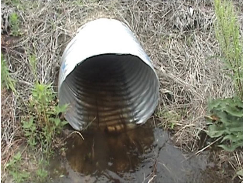
Sediment plume flowing into outfall pipe (May)
