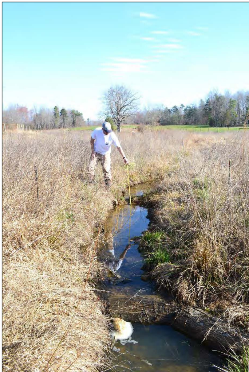
Photo 1: Substrate loss, 6" head-cut at UT 1, XC 9
