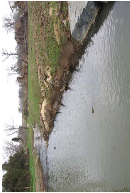
2. Bank Erosion: Moderate
