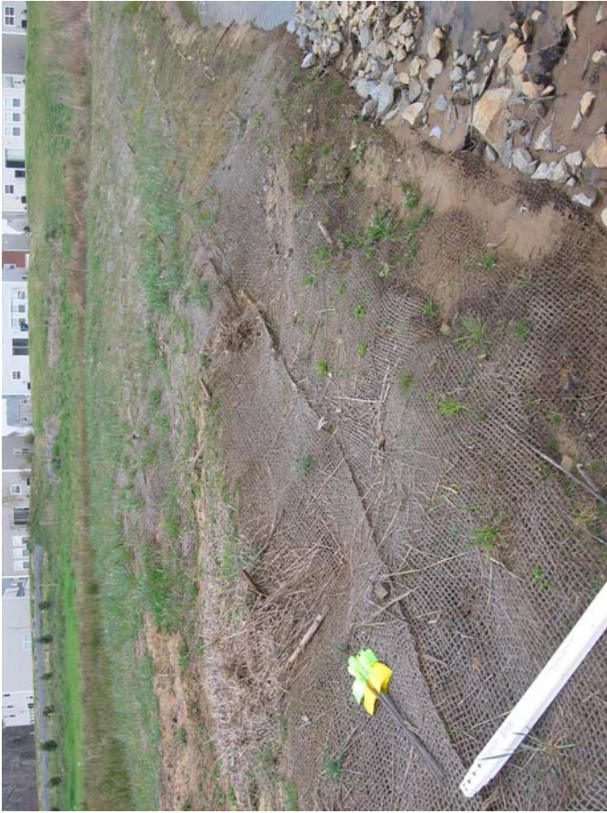
1. Bank Erosion - Moderate
