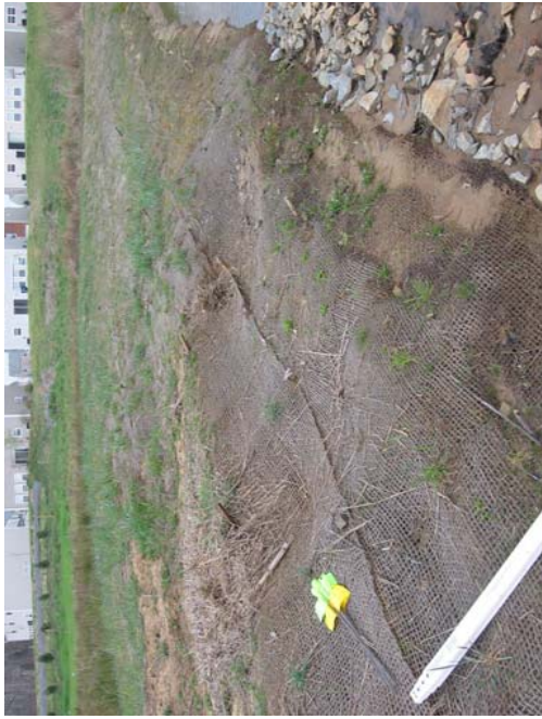
1. Bank Erosion: Moderate – Flood Event
