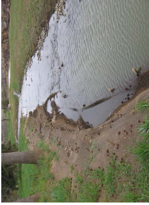
2. Loose matting – Flood Event
