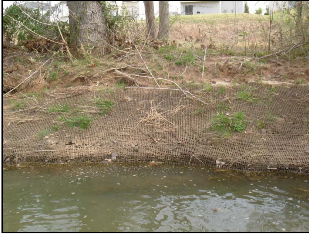
1. Bank Erosion: Moderate 3/22/2007
