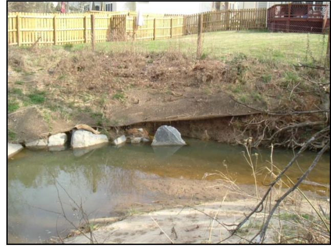
2. Bank Erosion: Severe 3/22/2007
