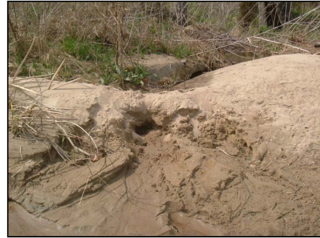
8. Heavy Sediment Deposition in Stormwater Swale 3/22/2007
