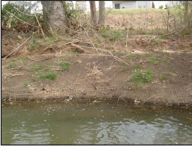
1. Bank Erosion: Moderate 3/22/2007
