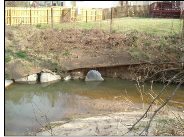
2. Bank Erosion: Severe 3/22/2007
