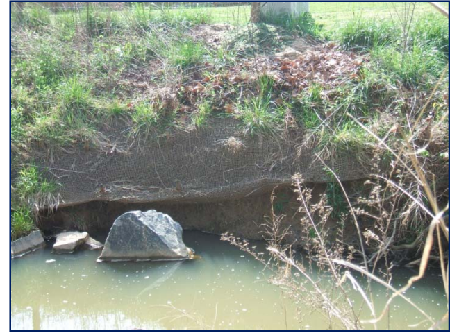
2. Bank Erosion: Severe (4/2008)
