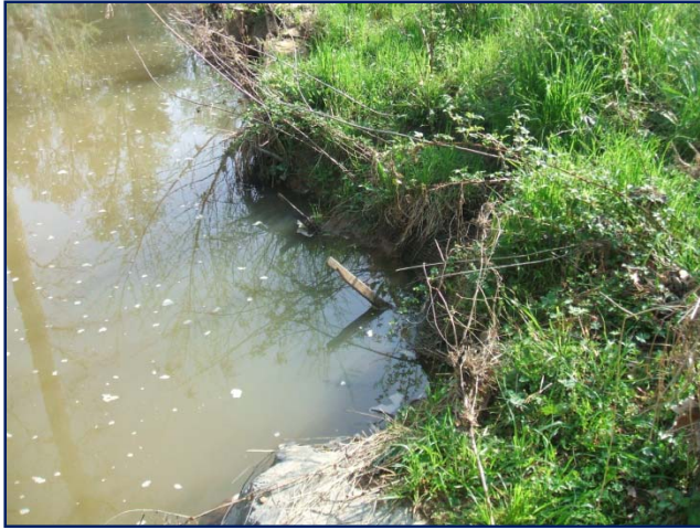
1. Bank Erosion: Moderate (4/2008)
