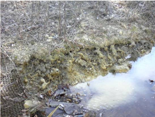
SPA 2. Bank scour.
