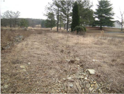
SPA 1. Stream overflow channel beginning to form.
