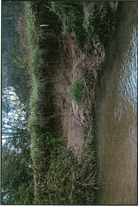
Photo 5 – Oct 04, Bank erosion at approximate proposed station 2+00, Upper Bailey
