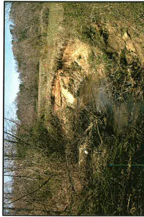
Photo 4 – Feb 04, Bank erosion at approximate proposed station 1+50, Upper Bailey
