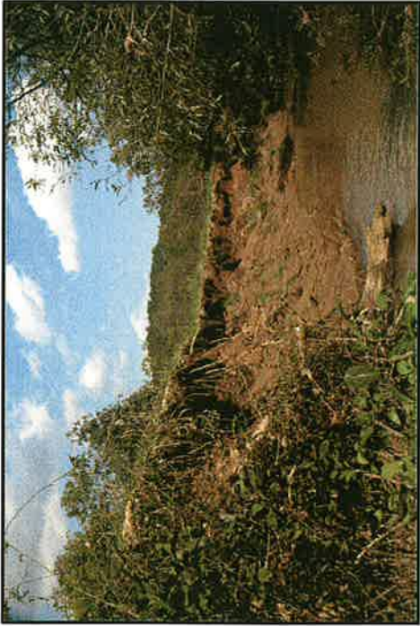
Photo 9 – Oct 04, Severe bank erosion, approximate proposed station 2+14, Lower Bailey
