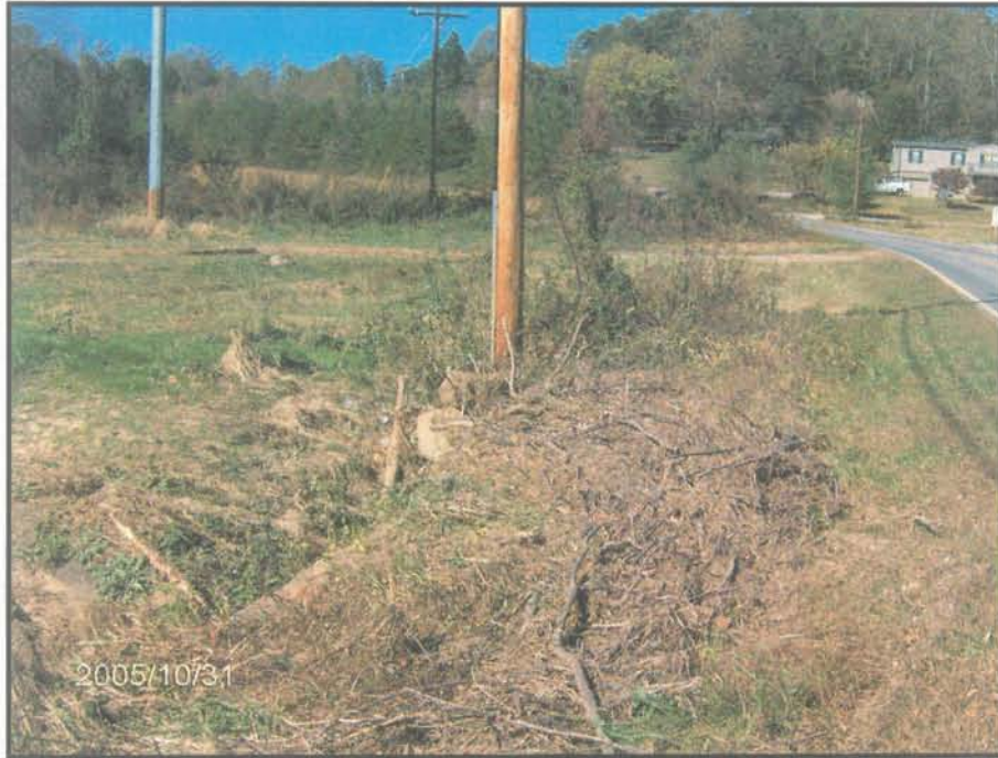
Photo 1 - Wrack line, Upper Bailey culvert headwall, photo date Oct. 31, 2005.
