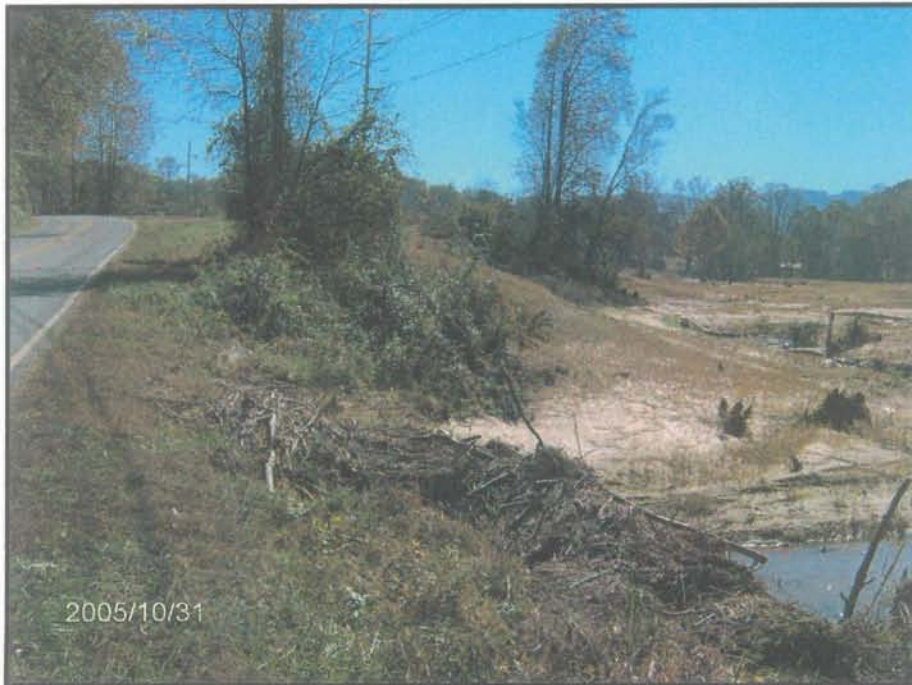
Photo 2 - Wrack line, Upper Bailey culvert headwall, photo date Oct. 31, 2005.
