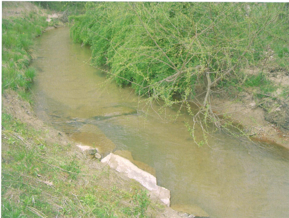
SPA 4 Stressed or failing structure along Upper Bailey Fork at station 1+25. Buried J-hook. (EMH&T, Inc. 4/13/07)
