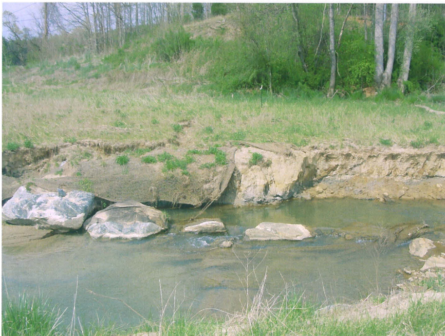
SPA 2 Bank failure along Upper Bailey Fork between stations 11+25 and 11+75. (EMH&T, Inc. 4/13/07)
