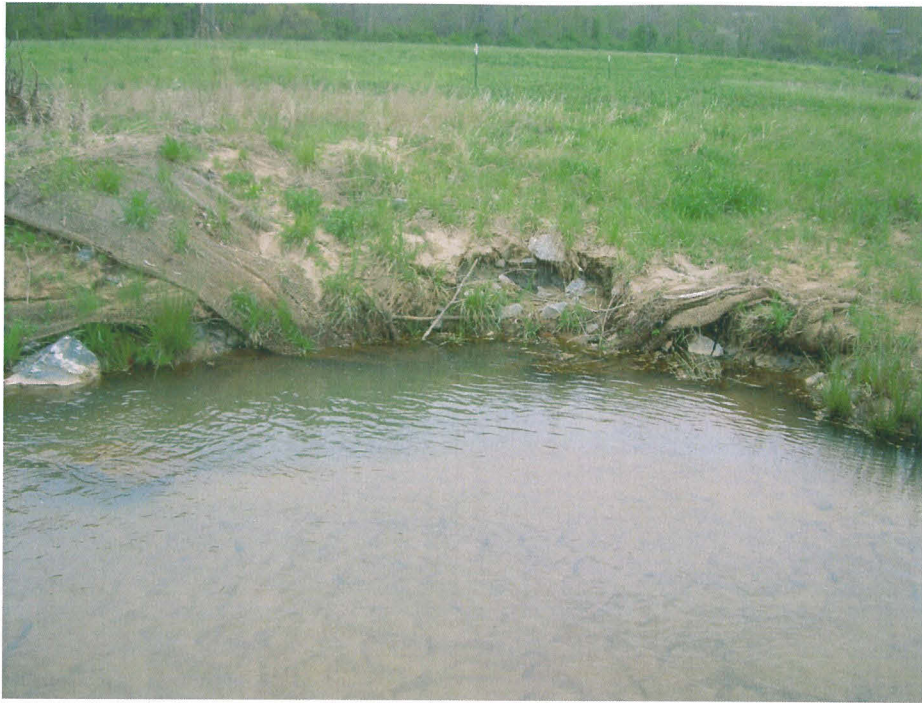
SPA 3 Bank scour along Upper Bailey Fork at station 3+50. (EMH&T, Inc. 4/13/07)
