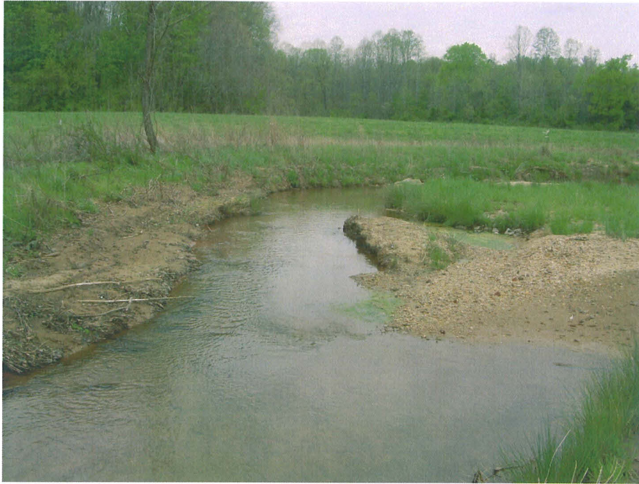
SPA 1 Area of aggradation along Upper Bailey Fork between stations 1+50 and 2+00. (EMH&T, Inc. 4/13/07)
