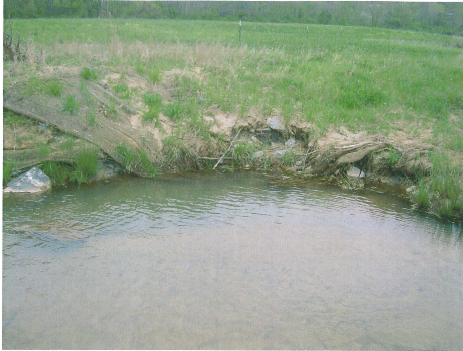
SPA 3 Bank scour in Year 1 along Upper Bailey Fork at station 3+50. (EMH&T, Inc. 4/13/07)
