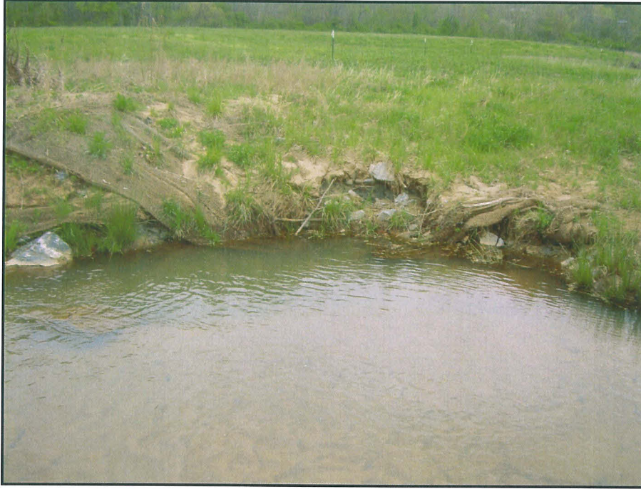
SPA 3 Bank scour in Year 1 along Upper Bailey Fork at station 3+50. (EMH&T, Inc. 4/13/07)
