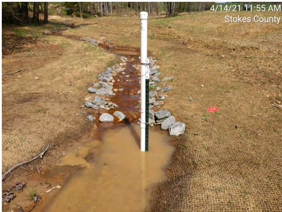
Crest Gauge CG-1 (UT2) Pressure Transducer
