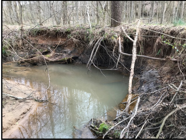
Looking at unstable conditions along BB-R3. Note the lateral bank erosion and lack of deep rooting vegetation.
