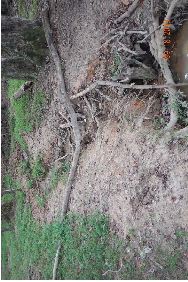
Reach UT2a – Erosion at headcut
