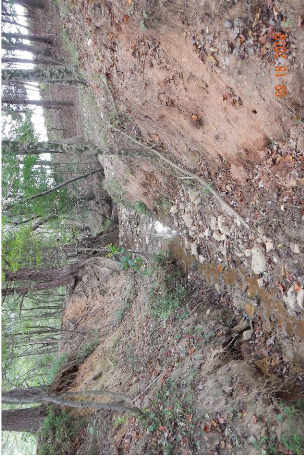
Reach UT2 – Incised and eroded channel
