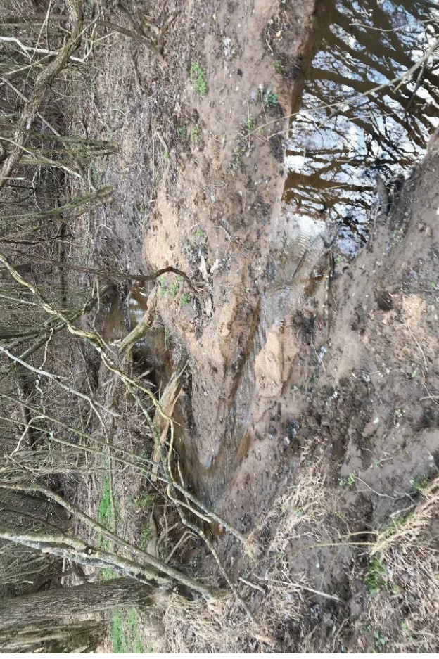
UT4-R2 – Minor bank erosion through W4
