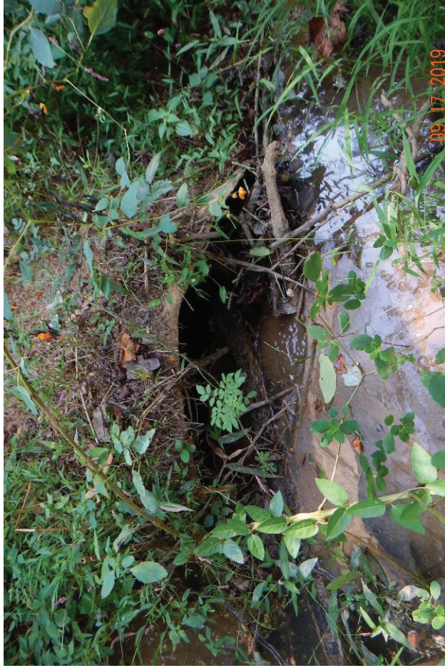
Reach UT1-R2 – Perched/Plugged culvert at farm crossing
