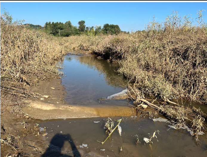
Pre-repair: BC R4b, STA 35+85, bank scour & structure issue (09/22/2022)
