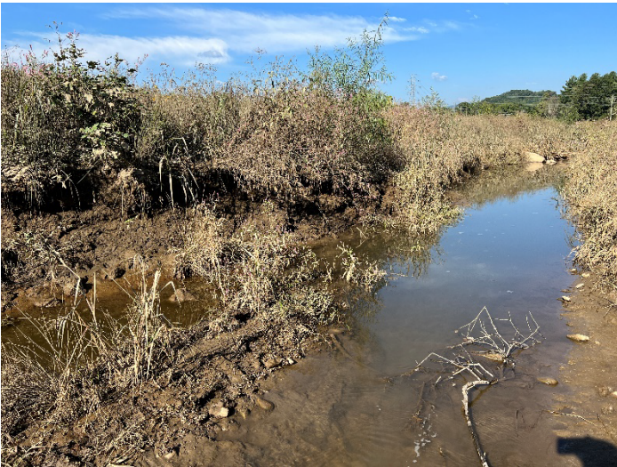
Pre-repair: BC R4b, STA 35+25, bank erosion and bed scour (09/22/2022)
