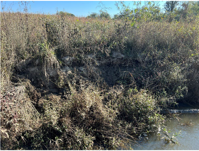
Pre-repair: BC R4b, STA 34+55, left bank erosion (09/22/2022)
