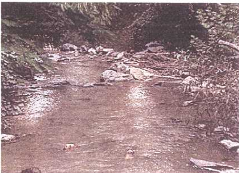
Site of the second vane, taken from the first vane downstream. Top photo shows site before construction, middle photo is the site during construction and bottom photo is three months after construction.
