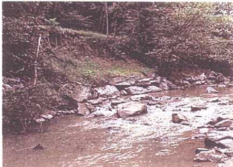
Bench construction at the lower end of the reach. Top photo shows the condition of the high vertical bank before construction. Middle photo shows construction and bottom photo shows site three months after construction.
