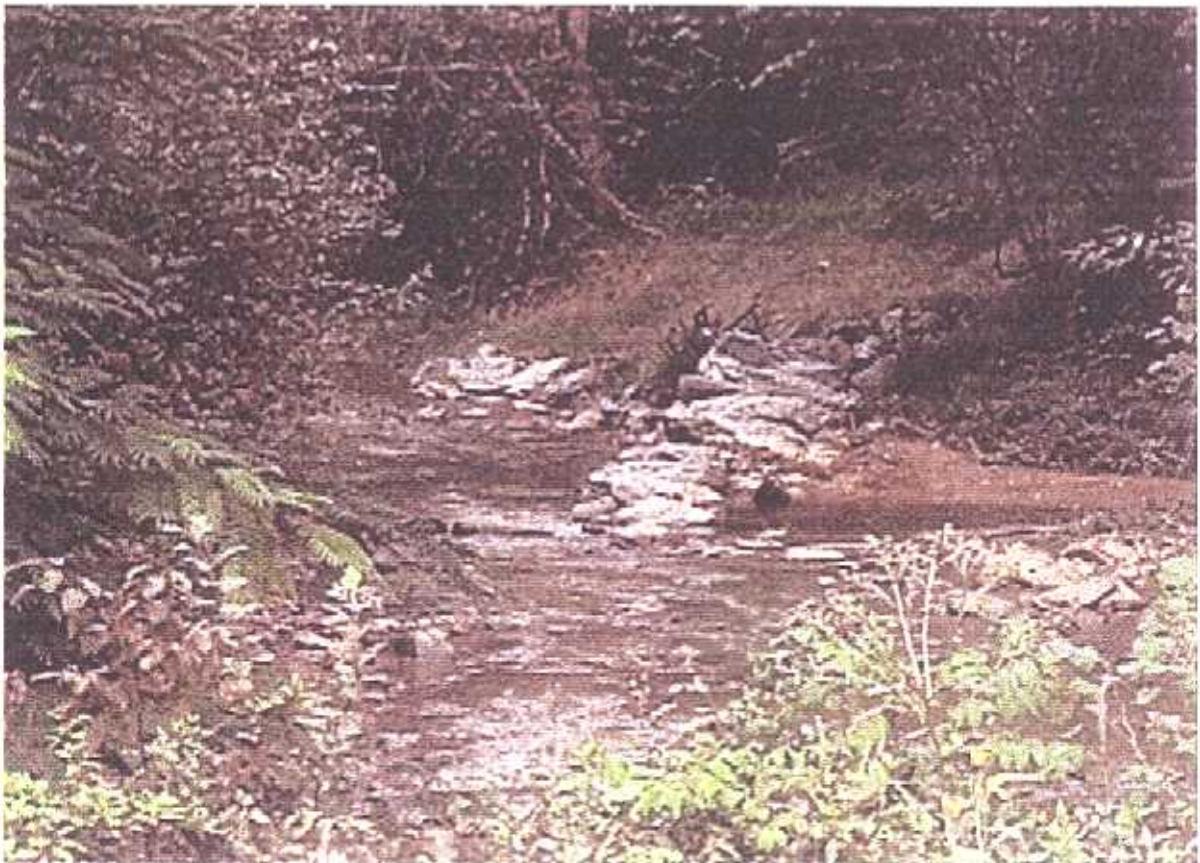
Upper photo - the third vane after construction showing high water pooling upstream of the vane and falling toward mid-channel. Bottom photo - shows the same vane with sediment deposited above the vane as water slows and the sloped, vegetated bank.
