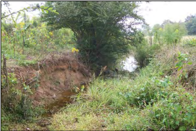
Photo 1-View of left bank erosion along Bear Creek Reach A, facing downstream.
