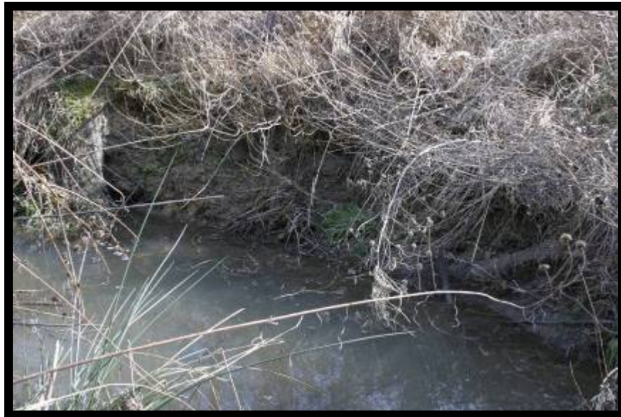
Station 09+40 Bank Slump
