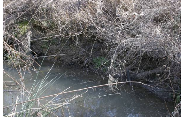
Issue Photo 2. Bank Erosion STA: 9+30
