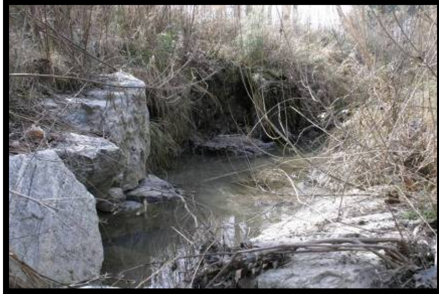
Station 01+60 Root Wad Vane Failure
