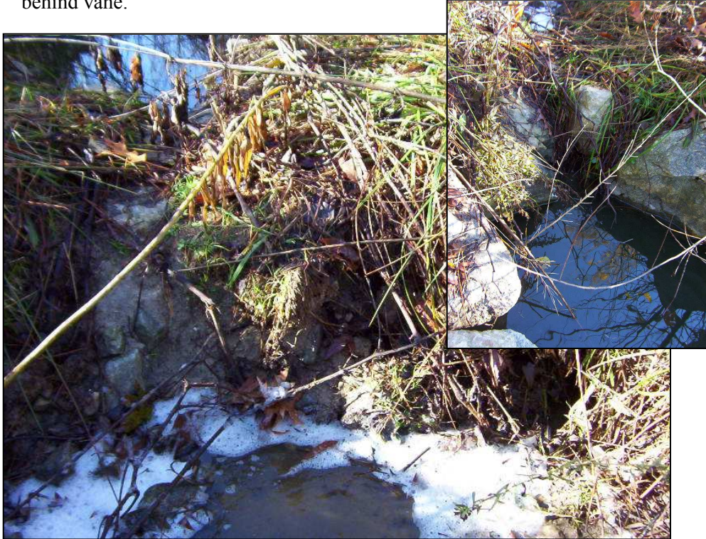
Photo 3. Piping of flow behind Rock Vane 3, causing moderate degradation of channel behind vane.
