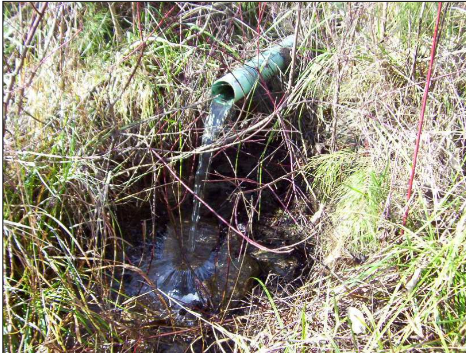
Photo 10. Erosion directly adjacent to stream from incoming 4-inch pipe.
