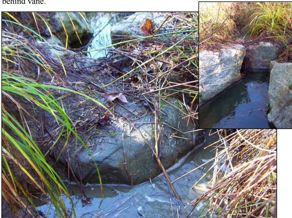
Photo 4. Piping of flow behind Rock Vane 3, causing moderate degradation of channel behind vane.
