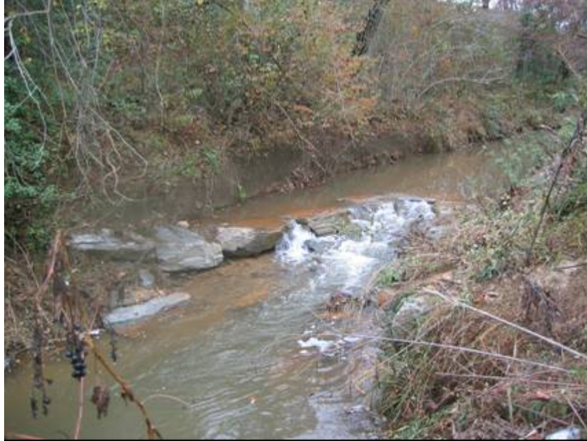
SP17. Station 20+10 to 20+40 Bank scour and erosion
