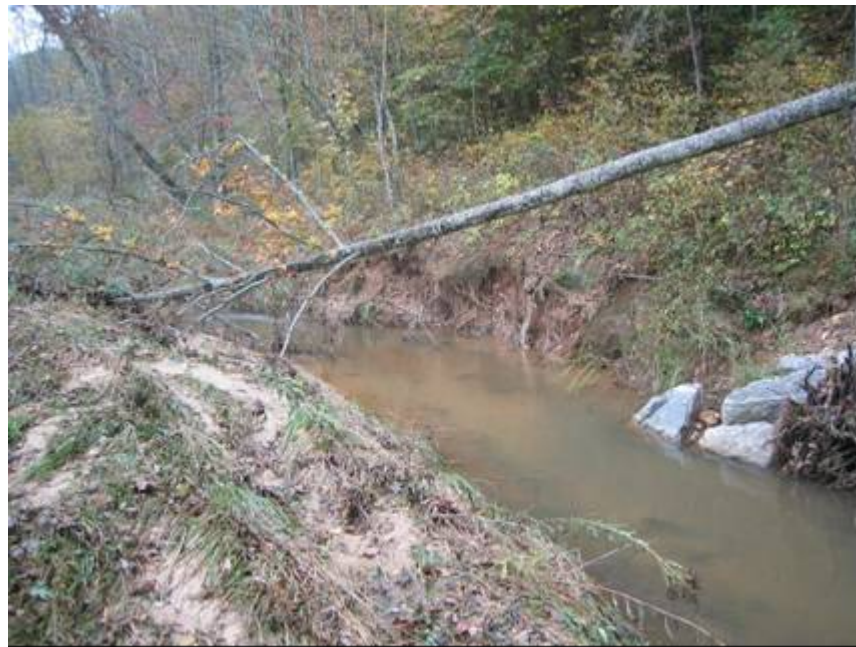
SP23. Station 28+90 to 29+10 Bank scour from debris jam
