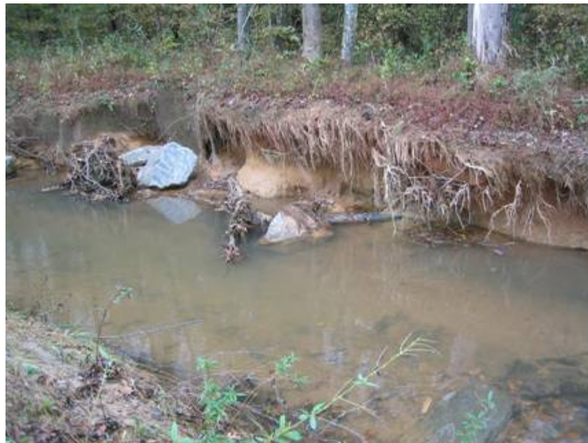
SP4. Station 8+80 to 9+20 Erosion and scour around root wads
