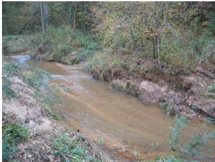
SP25. Station 35+40 to 35+80 Over wide
