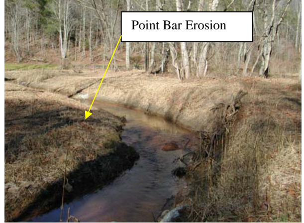
SP22. 2002 photo Station 27+10 to 27+20 Point bar scour
