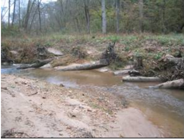
SP21. Station 27+10 to 27+20 Bank scour
