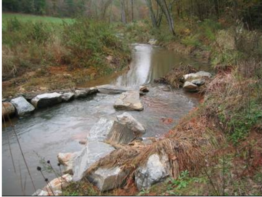
SP9. Station 12+00 to 12+60 Blowout around root wad and cross vane
