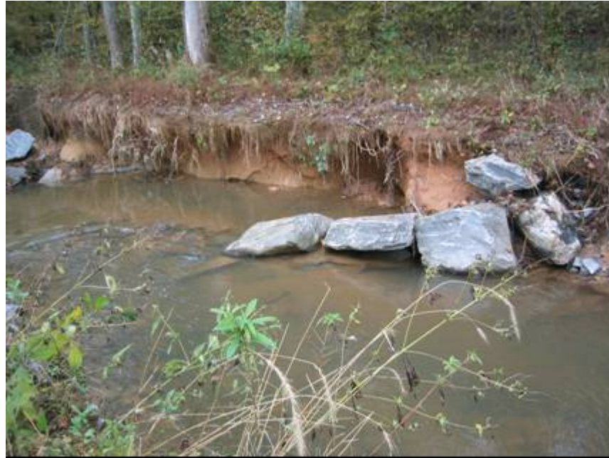
SP3. Station 8+80 to 9+20 Erosion and scour around root wads
