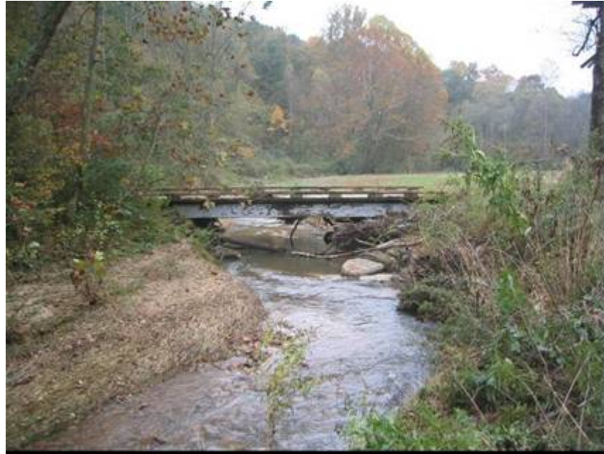
SP24. Station 30+50 to 31+00 Scour in front of root wad and bank erosion
