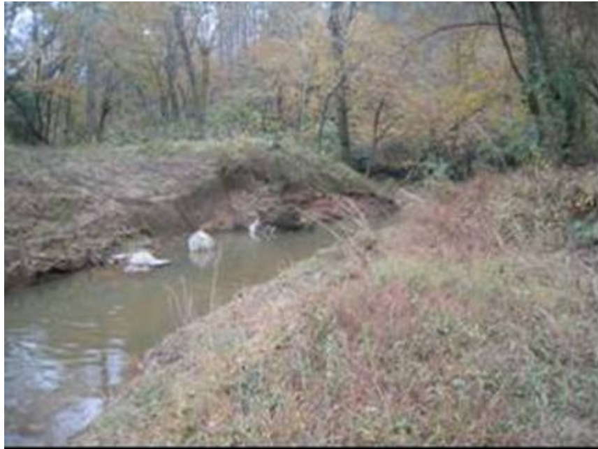
SP30. Station 42+00 to 42+30 Bank scour and bank slumping
