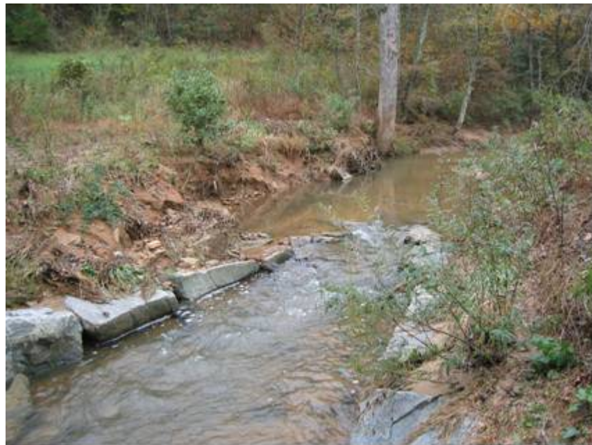
SP2. Station 8+10 to 8+30 Bank scour
