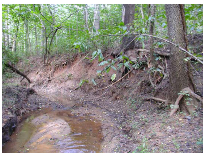
Photo 5 UT1 Bank Erosion
