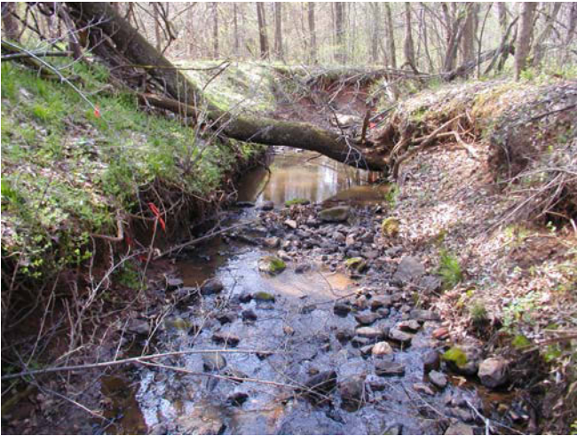
Photo 8 UT2 Bank Erosion
