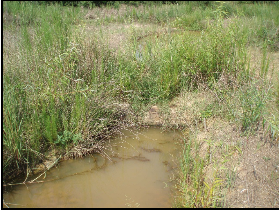
SPA 1. UT3B Sta. 316+00 Log weir set to high causing deposition and vegetation growth upstream.
