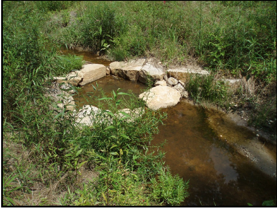
SPA 7. UT1A Sta. 134+60 Header rocks set to high at rock A-vane.
