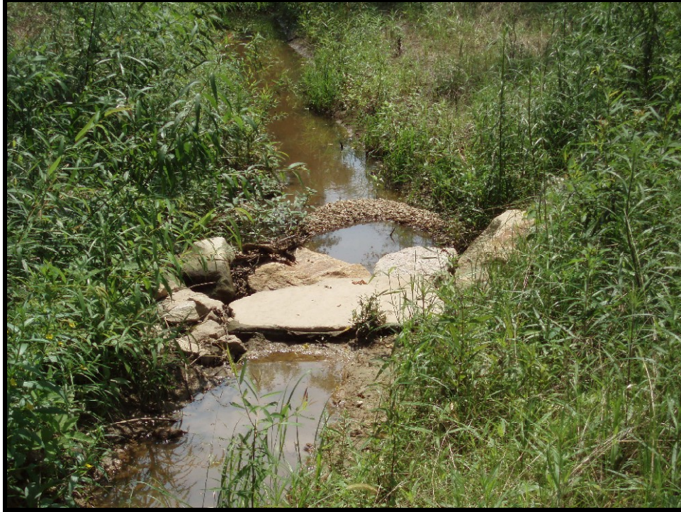
SPA 5. UT1A Sta. 133+40 Header rocks set to high at rock A-vane.
