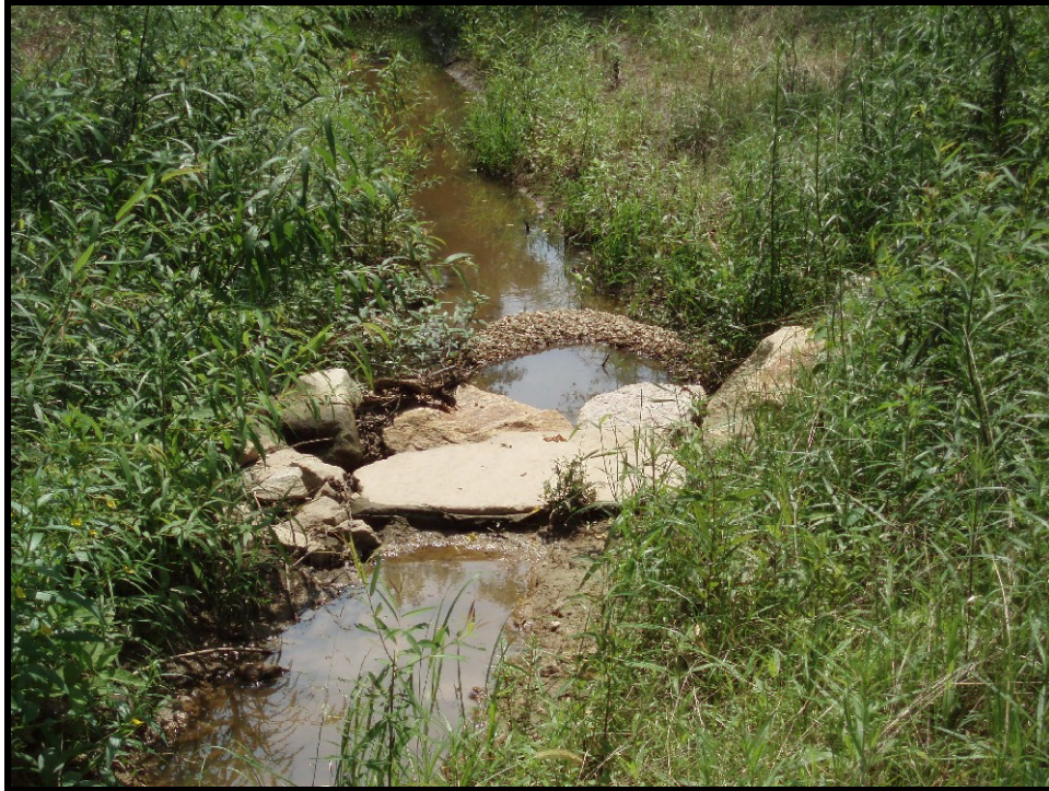
SPA5. UT1A Sta. 133+40. Improper installation of rock A-vane. Header rock set too high; stable but not functioning.
