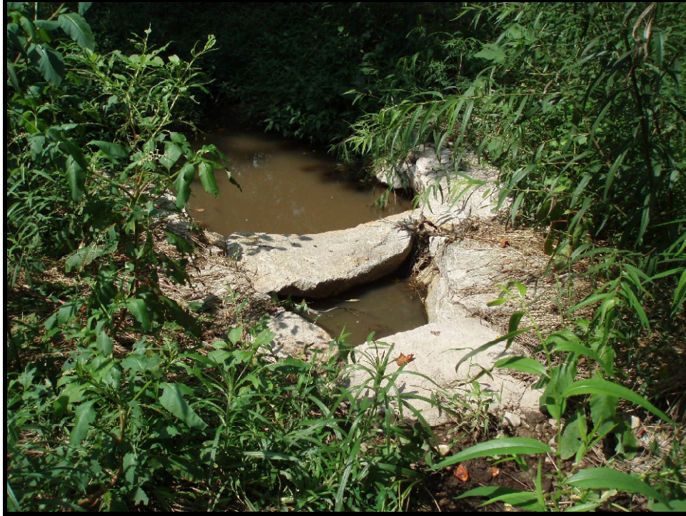
SPA3. UT2 Sta. 211+25. Erosion behind header rock of rock A-vane. Water flowing around both sides of header rock.
