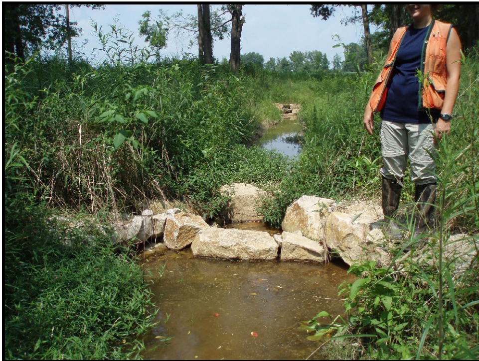
SPA 6. UT1A Sta. 134+00 Header rocks set to high at rock A-vane.
