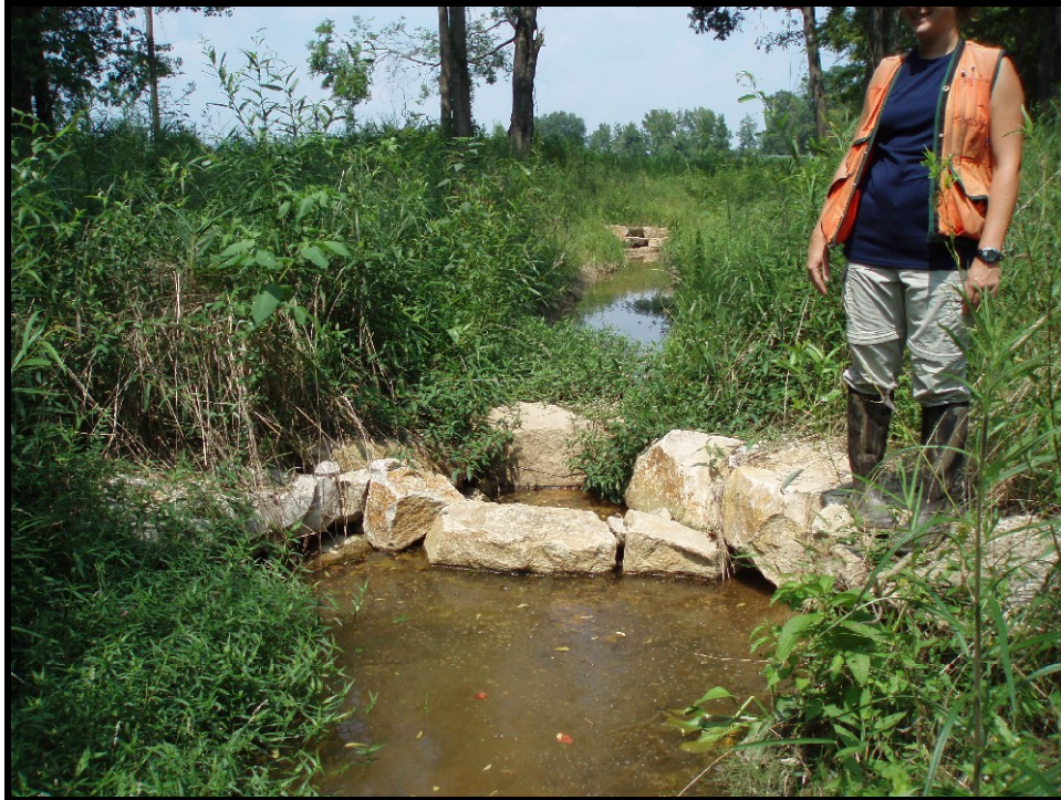
SPA6. UT1A Sta. 134+00. Improper installation of rock A-vane. Header rock set too high; stable but not functioning.
