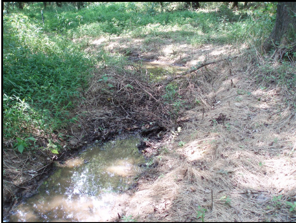
SPA 2. UT2 Sta. 203+80 Debris jam caused by fallen tree limbs and other woody vines.
