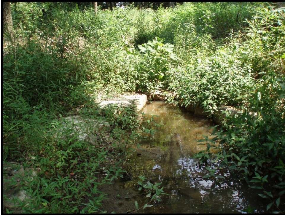
SPA4. UT2 Sta. 211+70. Improper installation of rock cross vane. Header rock set too high; water flowing around header rock.
