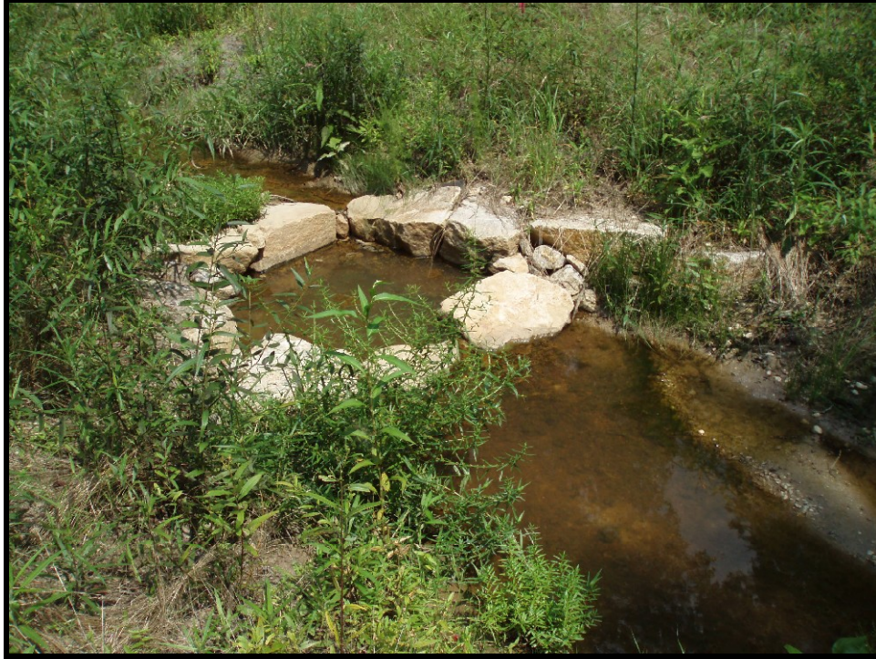
SPA7. UT1A Sta. 134+60. Improper installation of rock A-vane. Header rock set too high; stable but not functioning.
